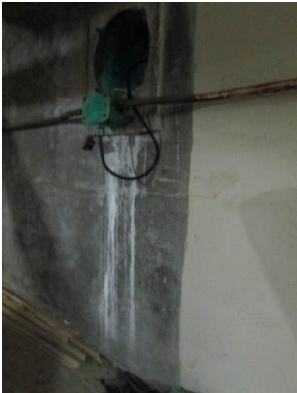
Image 11: Pool Leak at Light Niche
