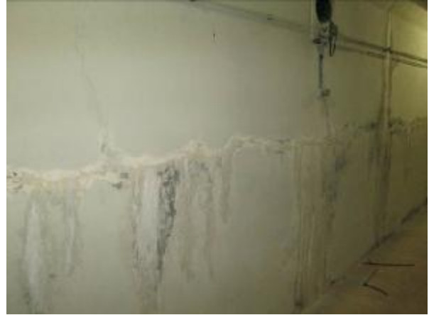
Image 8: Vertical Crack in the Pool Shell at the Interface of the Sloped Deep End Floor and the Pool Wall
