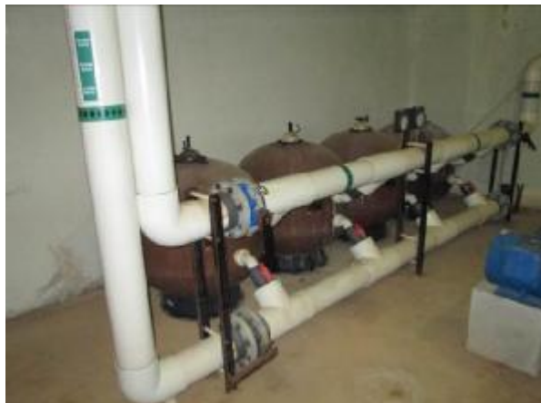
Image 84: High Rate Sand Filter Tanks
