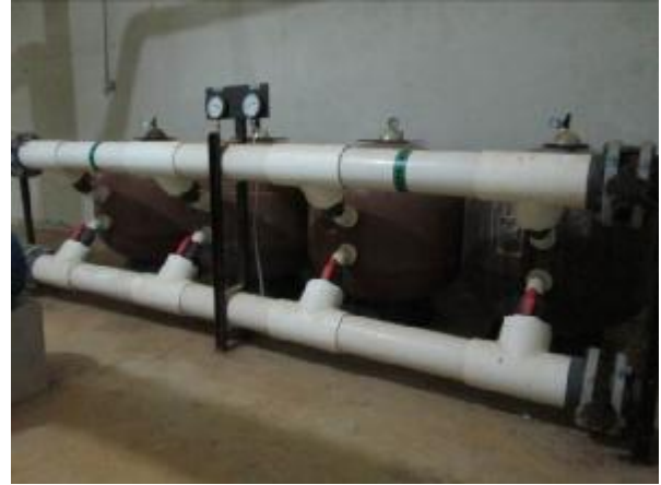
Image 87: Schedule 40 PVC Filter Face Piping
