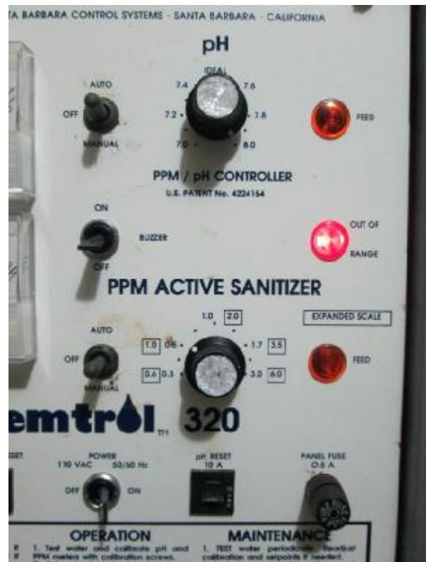
Image 108: Water Chemistry Controller Alarms and Controls
