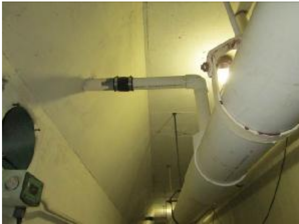
Image 70: Gutter Dropout Penetration
