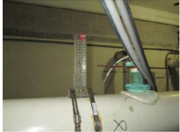
Image 75: Impact Flow Meter for Filtered Water Return
