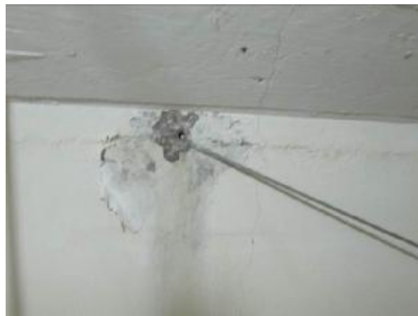
Image 65: Old Deck Plate Wiring at Shallow End
