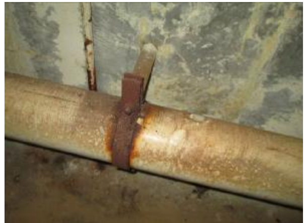
Image 73: Corroded Pipe Support
