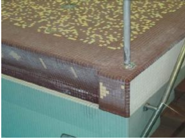
Image 15: Calcium Build-Up on the Rollout Gutter Curb above the Water Line
