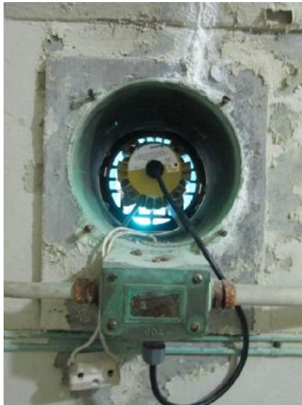
Image 29: Dry Niche and Backside of Underwater Light
