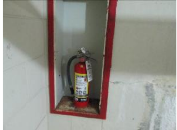
Image 18: ABC-type Fire Extinguisher in the Pool Tunnel Area
