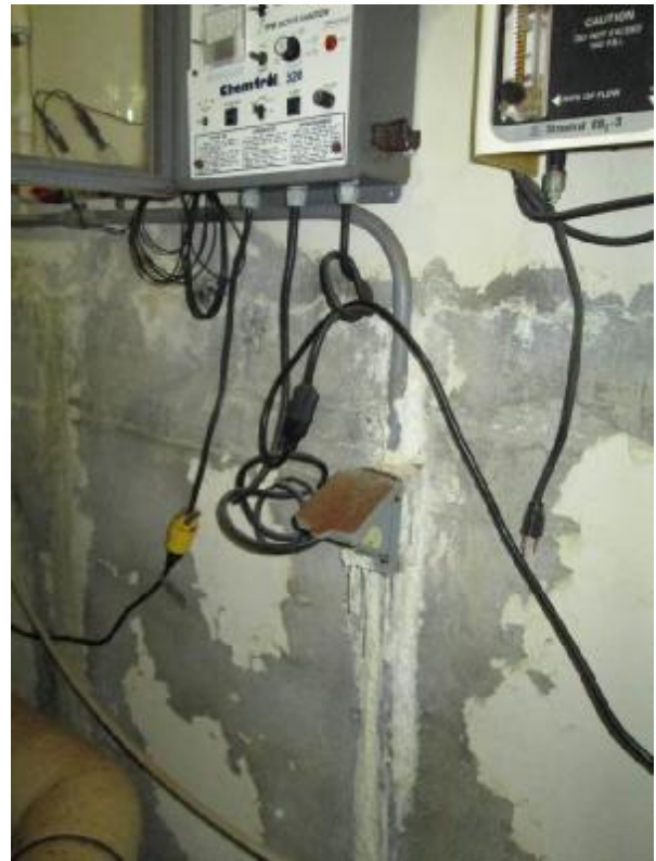
Image 110: Water Chemistry Controller Wiring Connections
