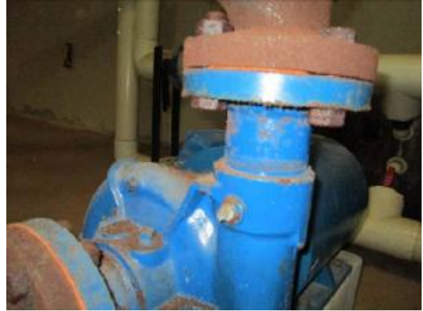
Image 81: Pump Tap for Pressure Gauge
