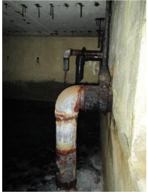
Image 112: Domestic Water Coming into Surge Tank
