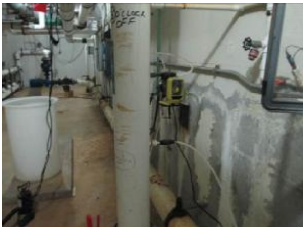
Image 96: Pool Chemical Feed Location
