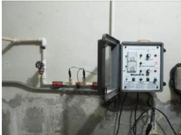
Image 109: Water Chemistry Controller and Probes
