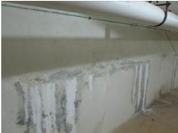
Image 9: Crack in the Pool Structure
