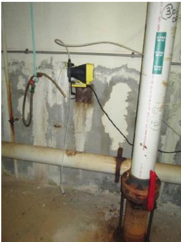
Image 100: Chemical Feed Pump
