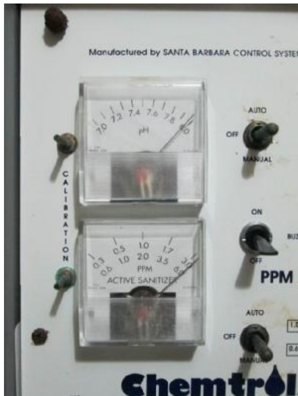
Image 107: Water Chemistry Controller Meters
