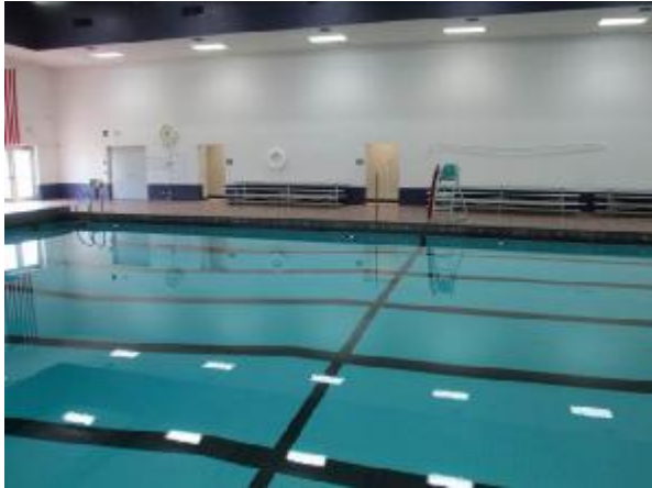
Image 27: Swimming Pool Underwater Lighting
