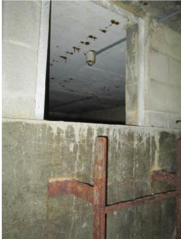
Image 94: Surge Tank Access and Ladder
