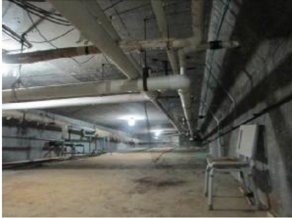
Image 68: Piping and Hangers near Surge Tank
