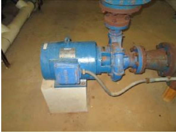
Image 80: Recirculation Pump and Base
