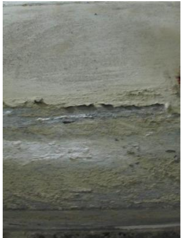
Image 2: Crack in the Pool Structure
