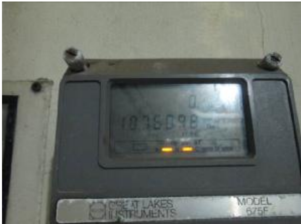
Image 76: Digital Flow Meter
