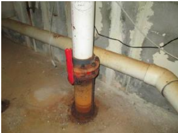
Image 72: Return Piping and Valve
