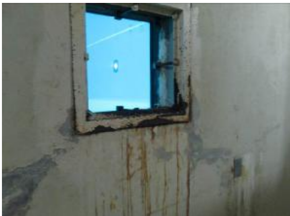
Image 19: Corrosion and Cracks around the Underwater Pool Window
