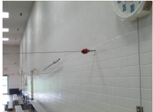
Image 52: Anchor Connection for Backstroke Cable
