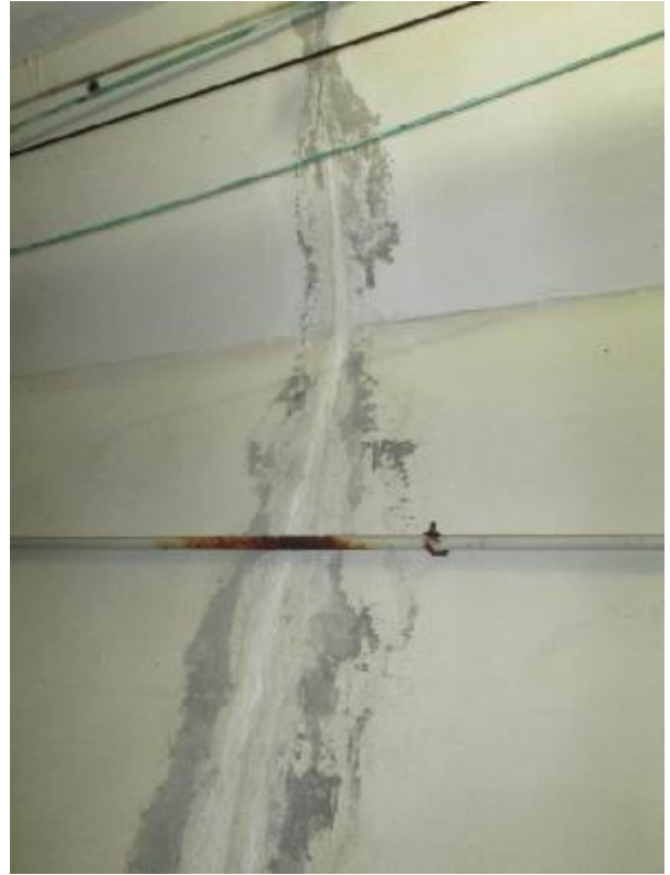
Image 4: Vertical Crack in the Pool Structure
