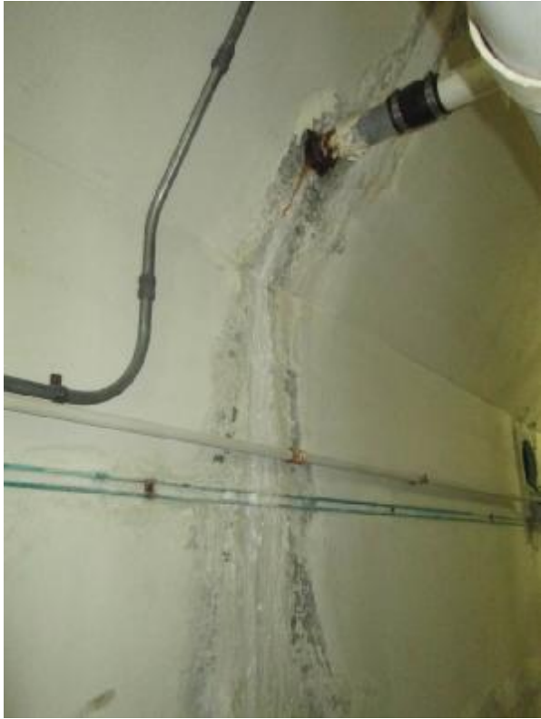
Image 3: Pool Leak Emanating from Pool Piping
