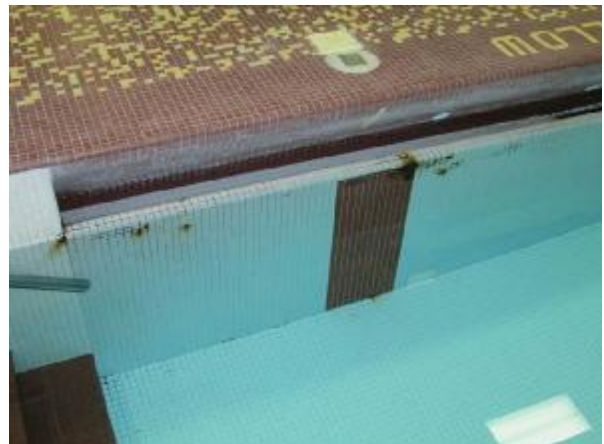
Image 14: Corrosion at the Water Line Handhold
