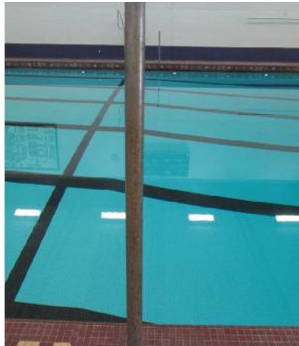
Image 53: Corrosion on Stanchion Post
