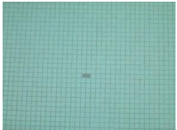
Image 12: Missing Tiles in the Shallow End
