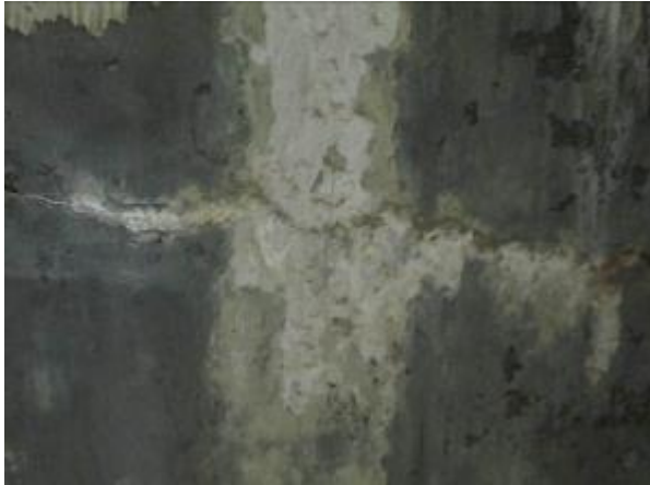
Image 5: Crack in the Pool Structure
