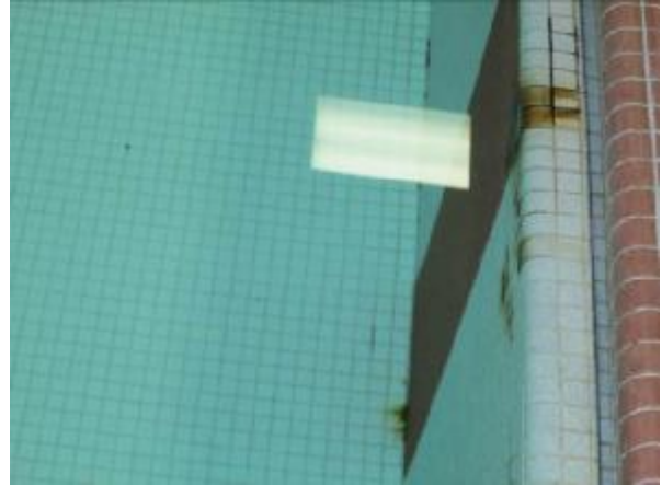
Image 16: Corrosion at the Water Line Handhold
