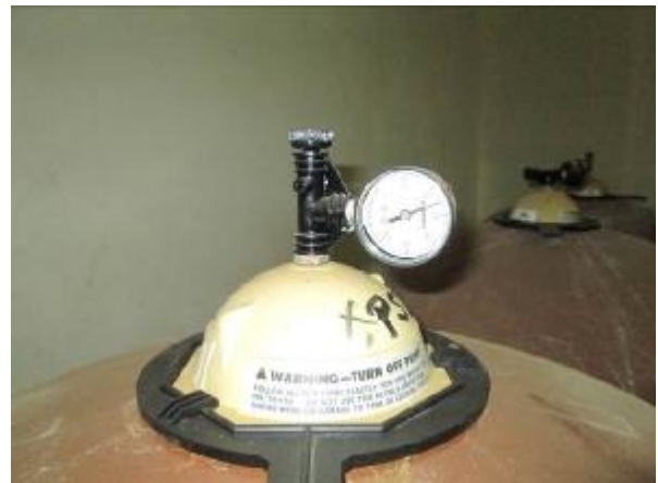
Image 85: Filter Tank Pressure Gauge
