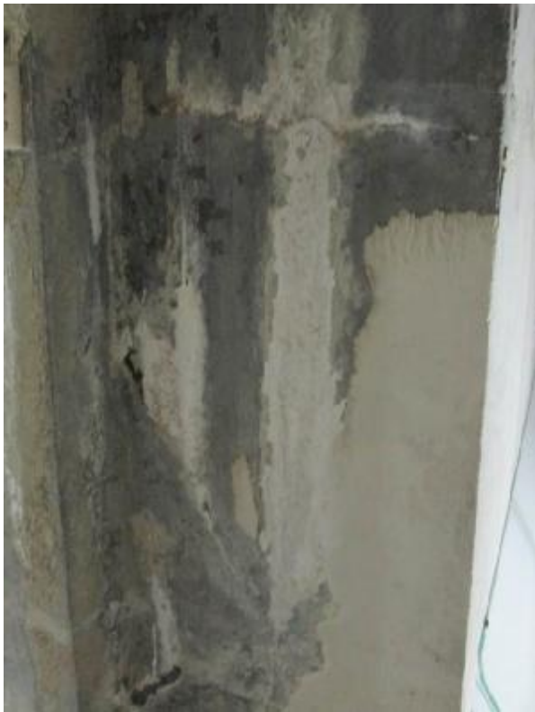
Image 1: Crack in the Pool Structure
