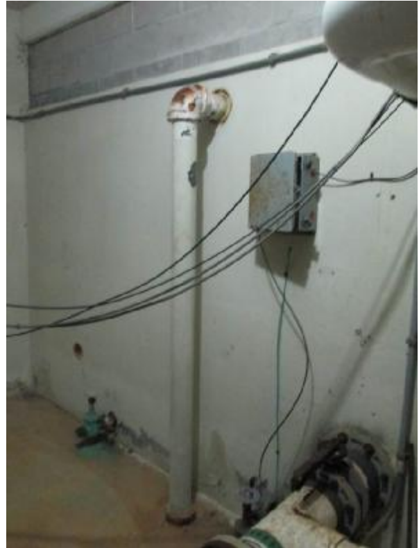
Image 95: Surge Tank Overflow
