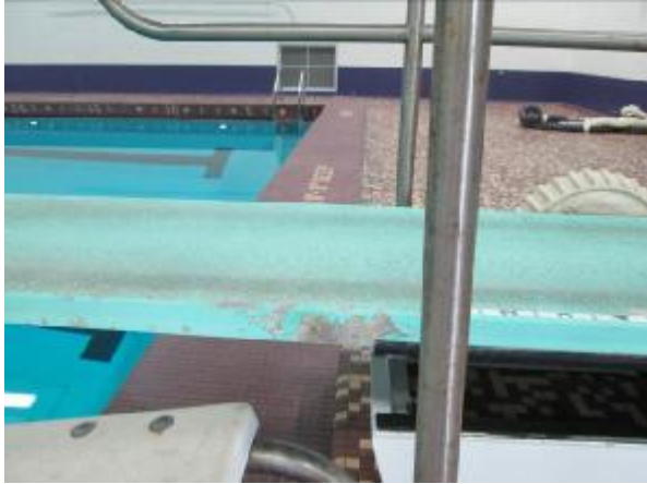
Image 46: Delamination of Diving Board Board
