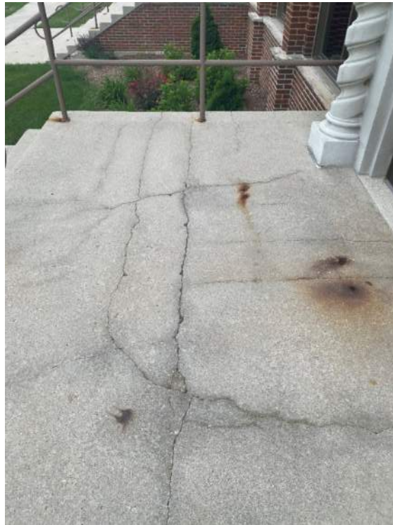
Figure 9: Top of center east concrete stairs in poor condition.
