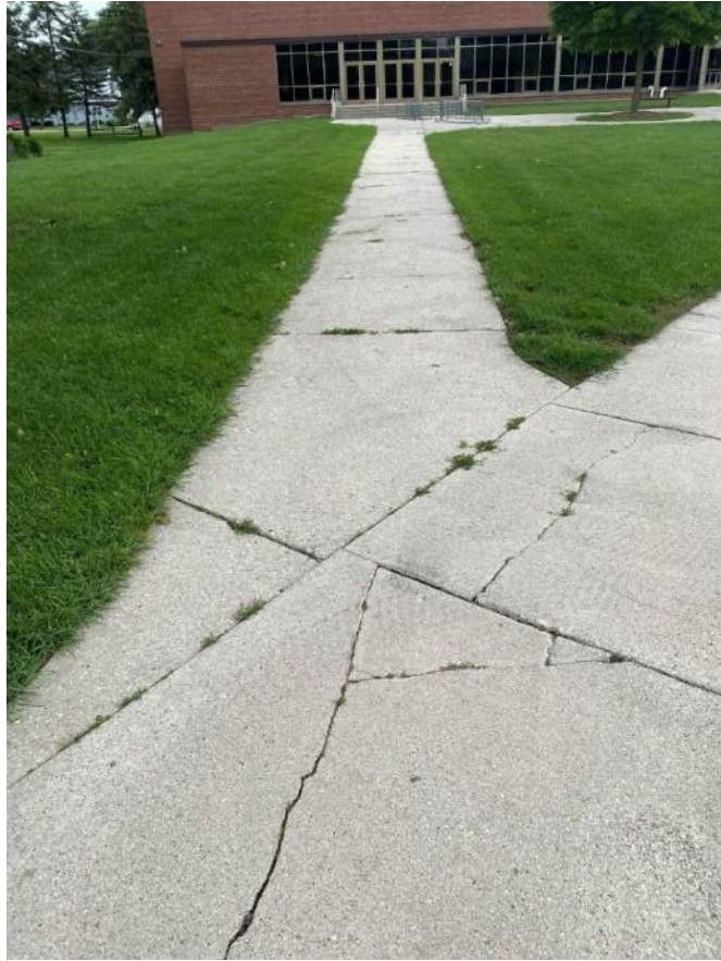
Figure 28: Cracking in front west sidewalk.
