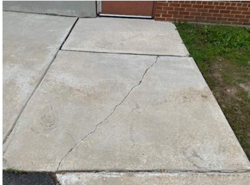
Figure 33: Cracked concrete slab at west door on back side of school.
