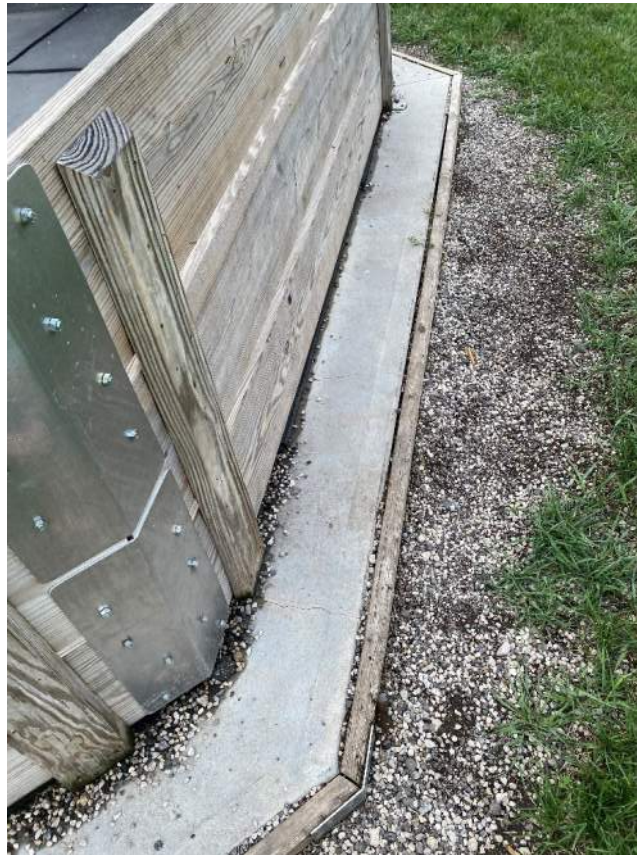
Figure 57: Cracks in concrete base for wooden octagon.
