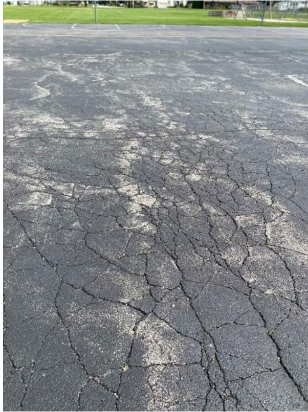
Figure 41: Severe alligator cracking in back play yard.
