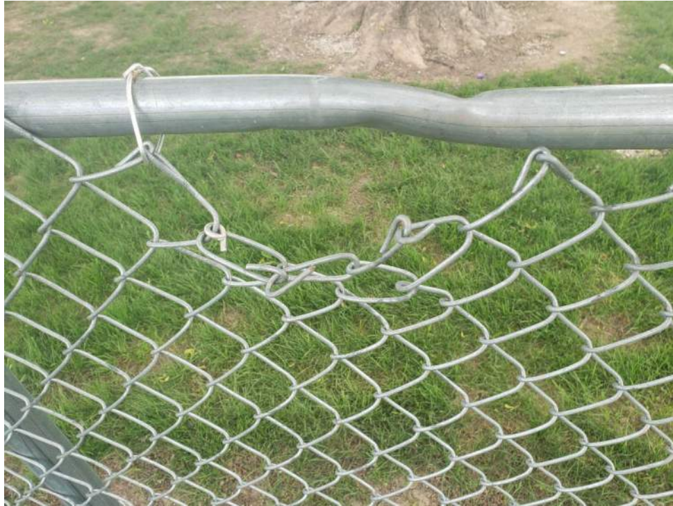
Figure 23: Broken links in the fencing that must be repaired/replaced
