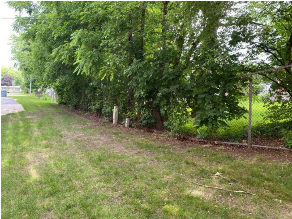
Figure 61: Metal fence on east property line falling over and overgrown with trees.
