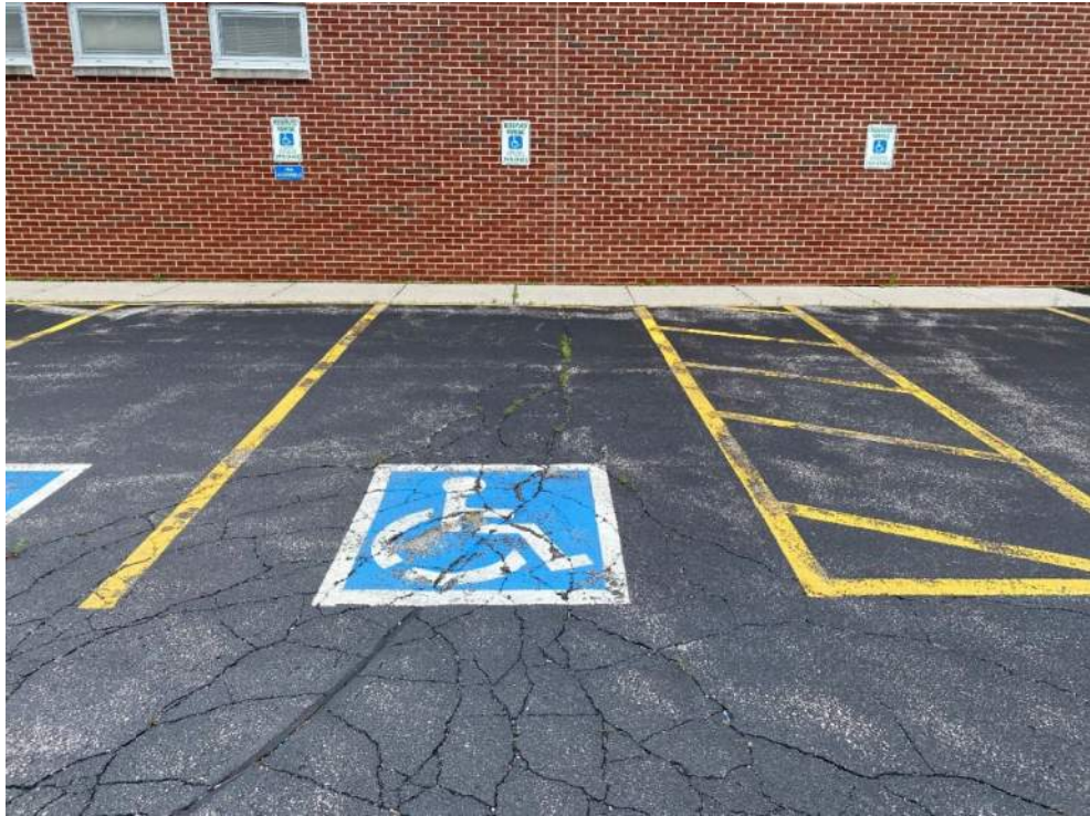
Figure 49: Alligator cracking in ADA stalls on east side of back of school.
