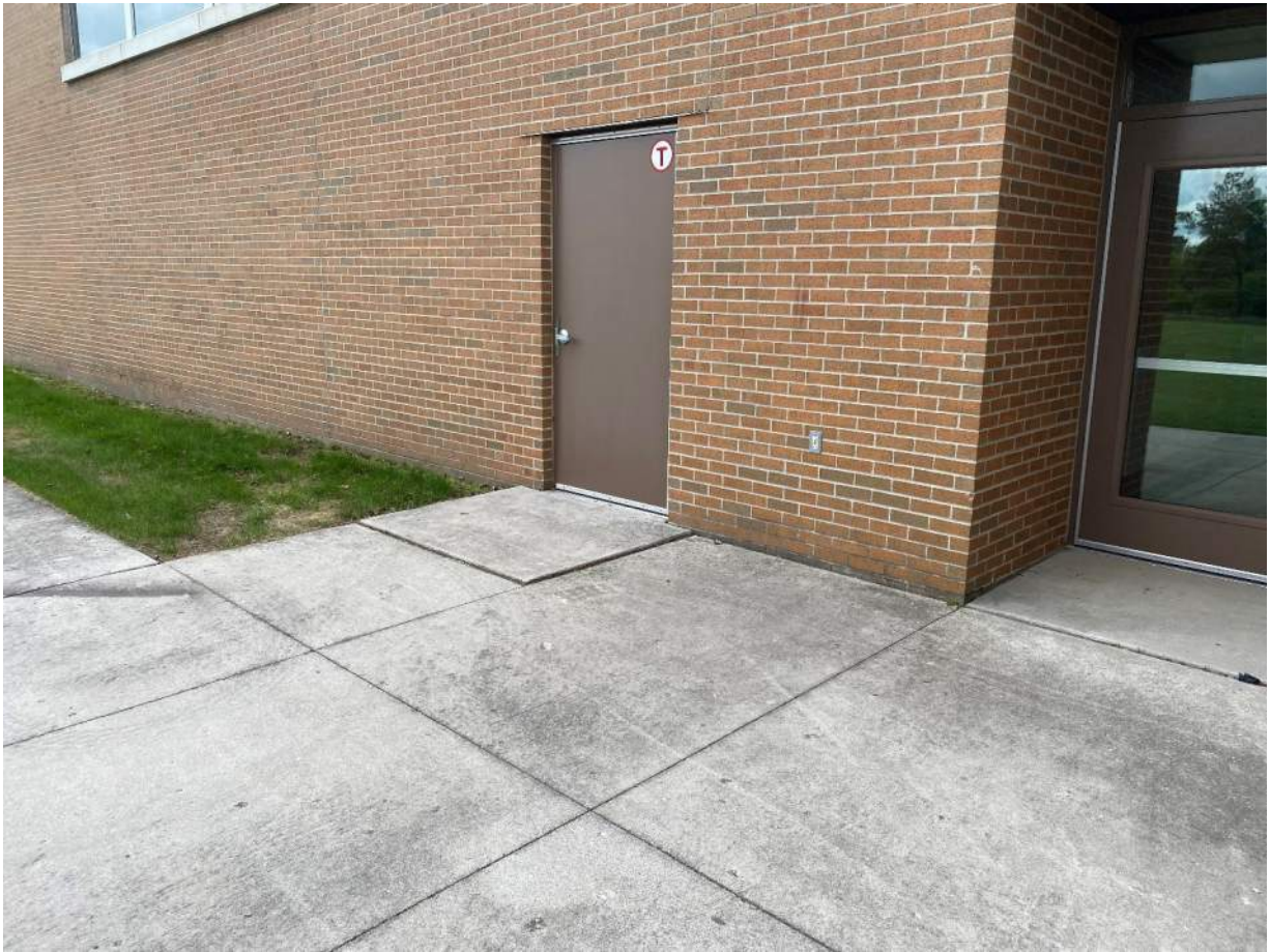
Figure 20: Worn sidewalk and stoop height higher than surrounding pavement on north side of school
