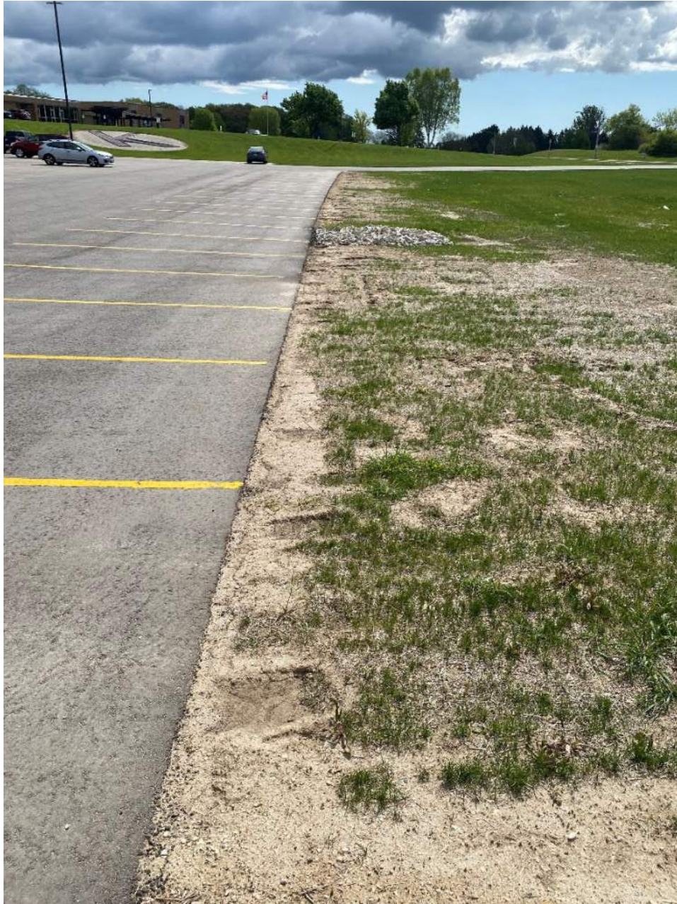
Figure 10: Erosion and dead grass on south end of PAC Parking
