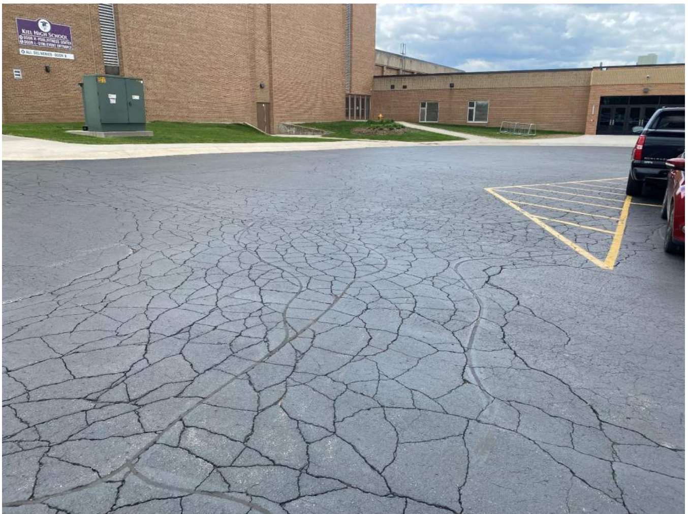
Figure 14: Alligator cracking in Student Parking Lot
