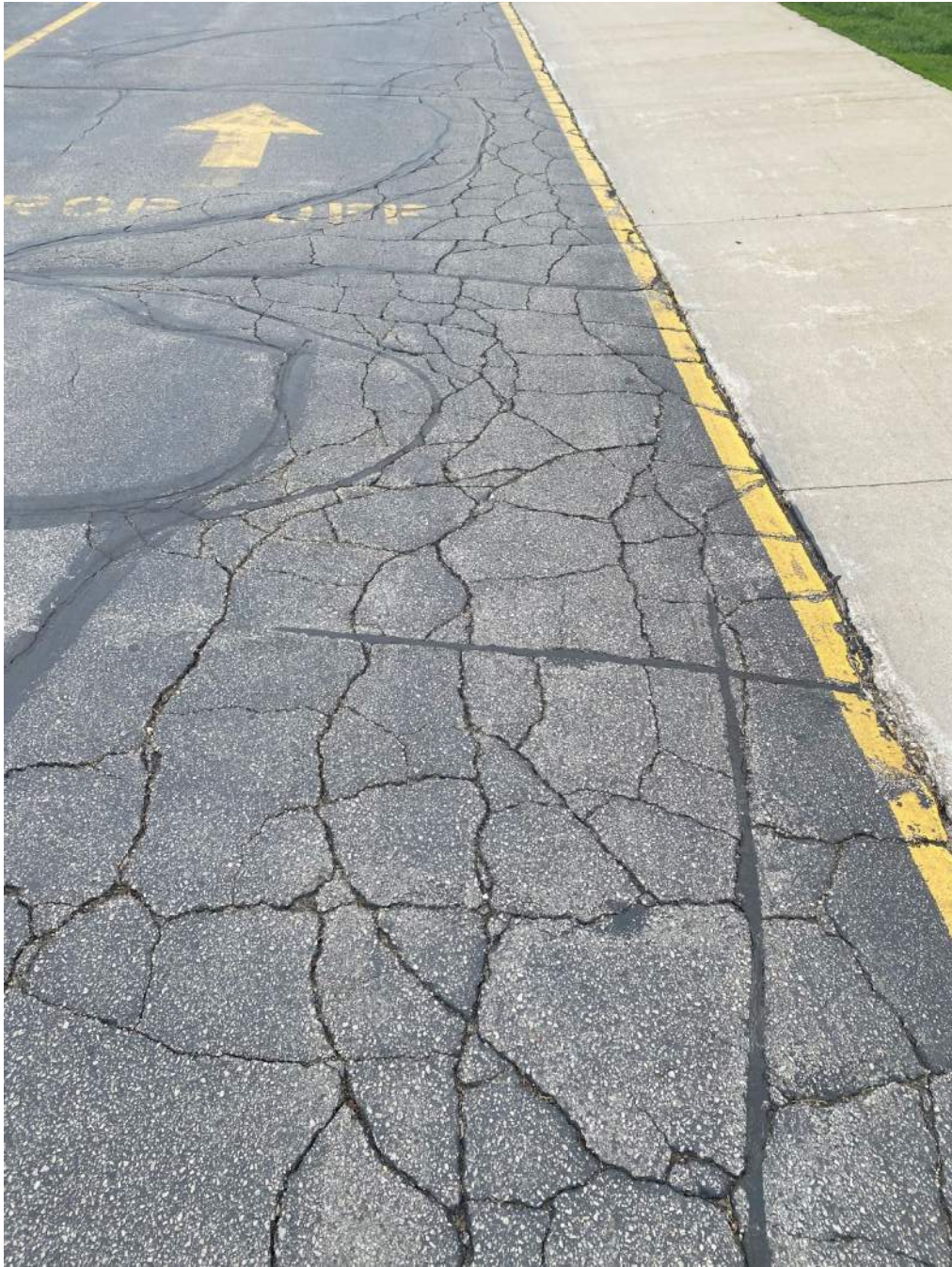
Figure 8: Alligator cracking in east driveway in south parking lot
