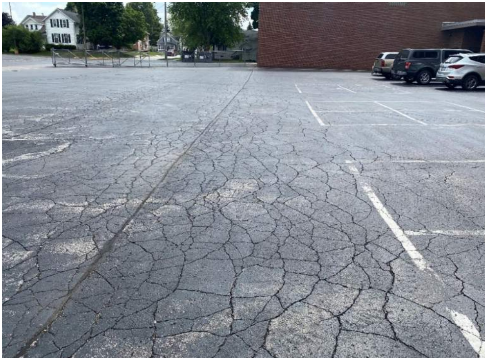
Figure 42: Alligator cracking throughout back play yard.
