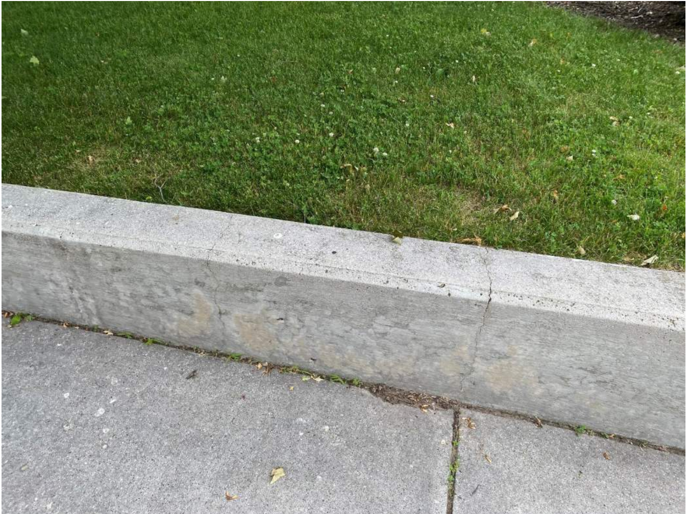
Figure 40: Cracking in concrete retaining wall in courtyard.
