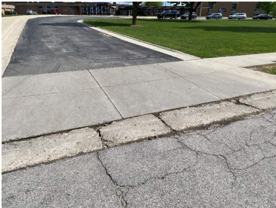
Figure 5: Cracked curb and gutter at exit driveway in Bus/Visitor Parking Loop.
