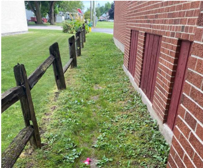
Figure 32: Wood fence on west side of school in poor condition.
