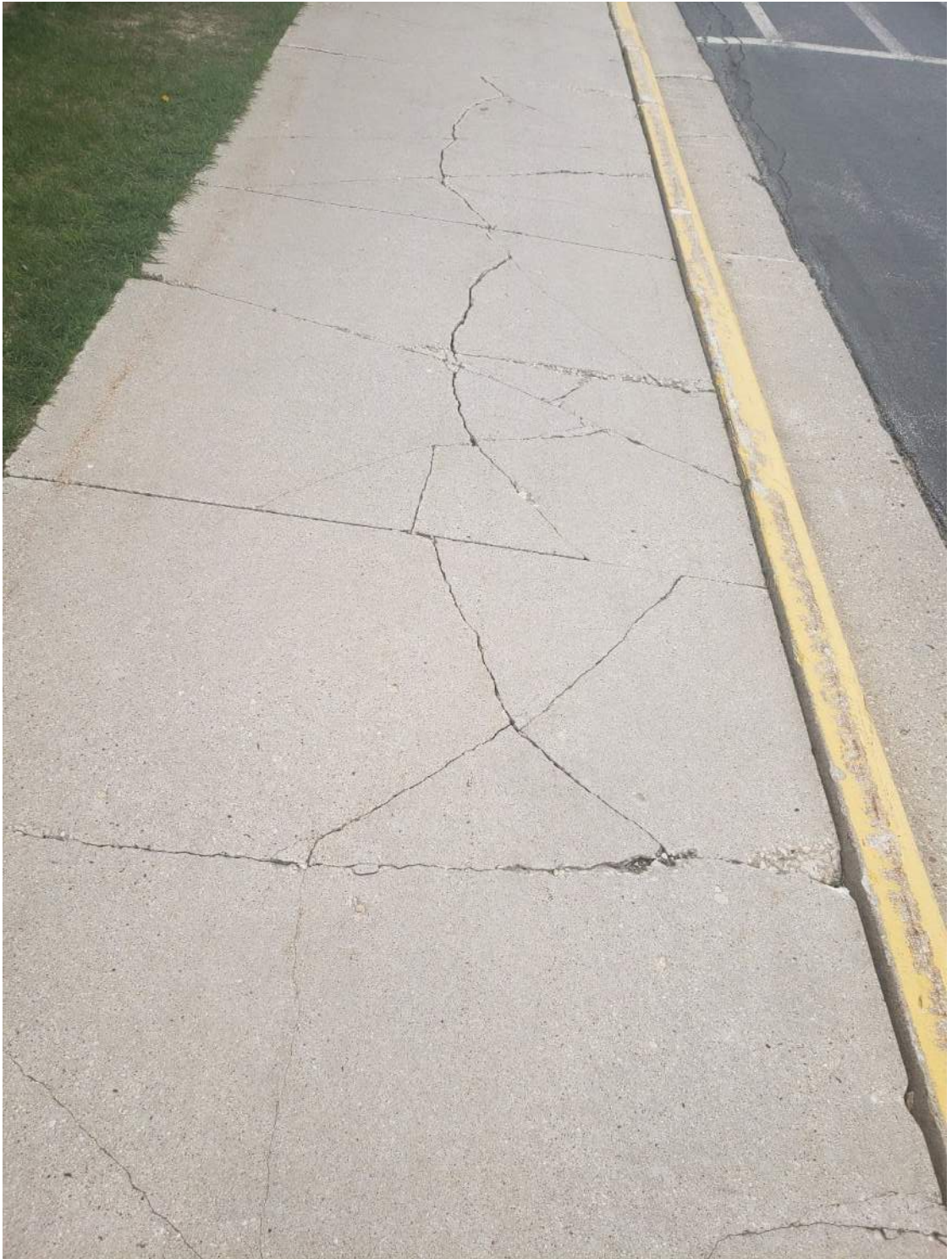
Figure 5: Severe cracking in sidewalk by north doors on west side of school.
