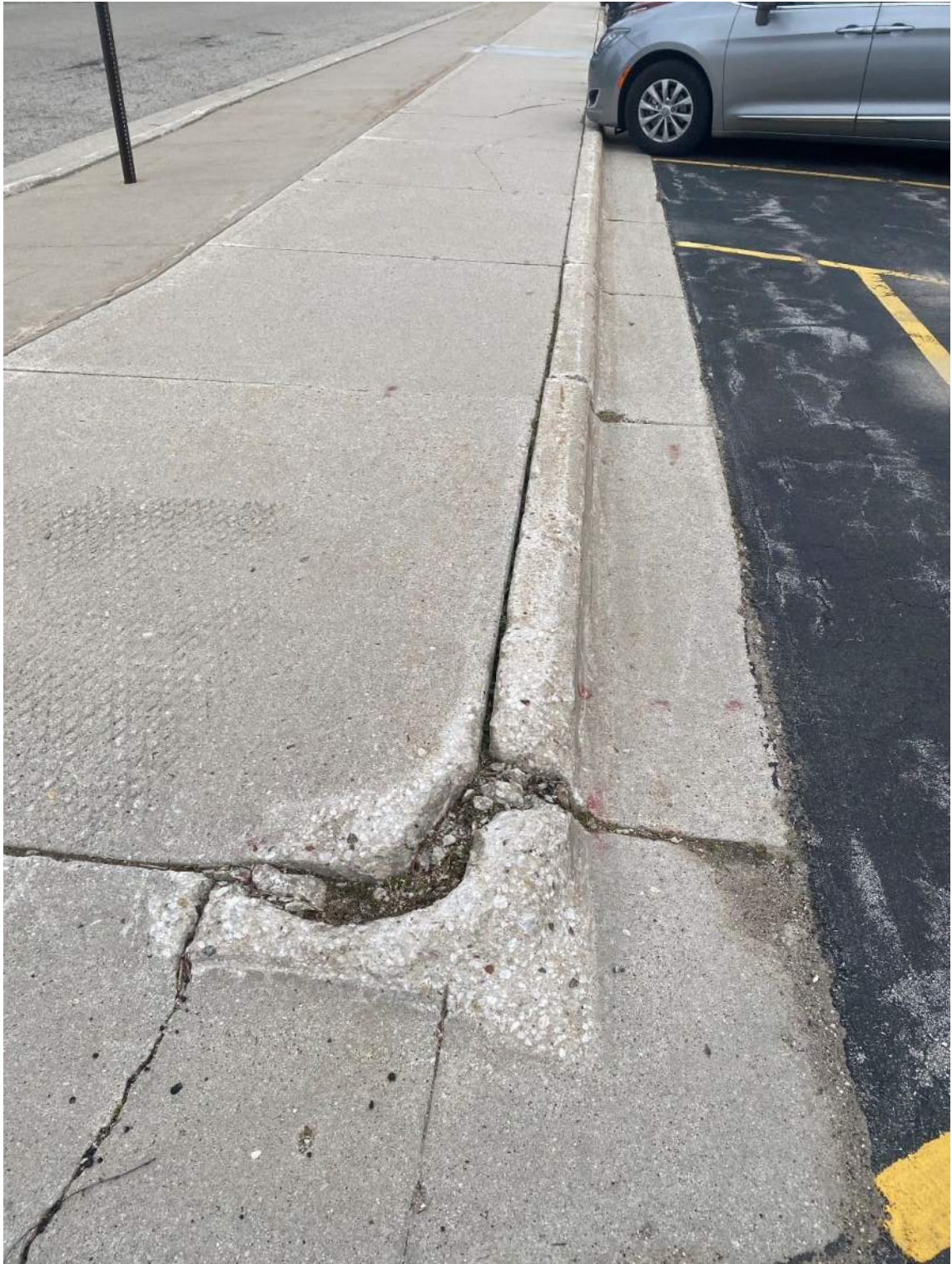
Figure 6: Deteriorated curb near south-west driveway apron
