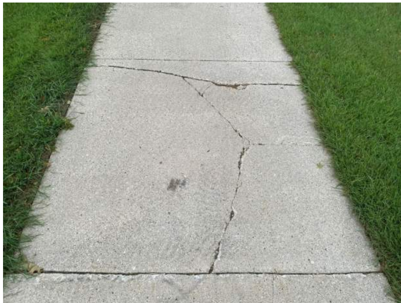
Figure 27: Additional cracking in front west sidewalk.
