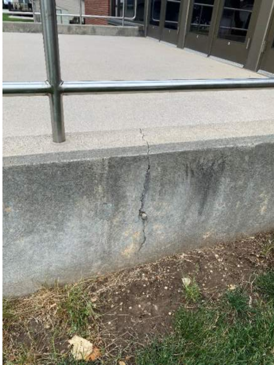
Figure 23: Crack in foundation of front west stairway.
