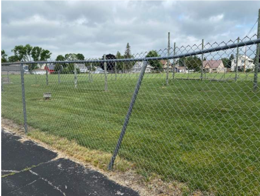
Figure 54: Fence surrounding climbing area falling over.
