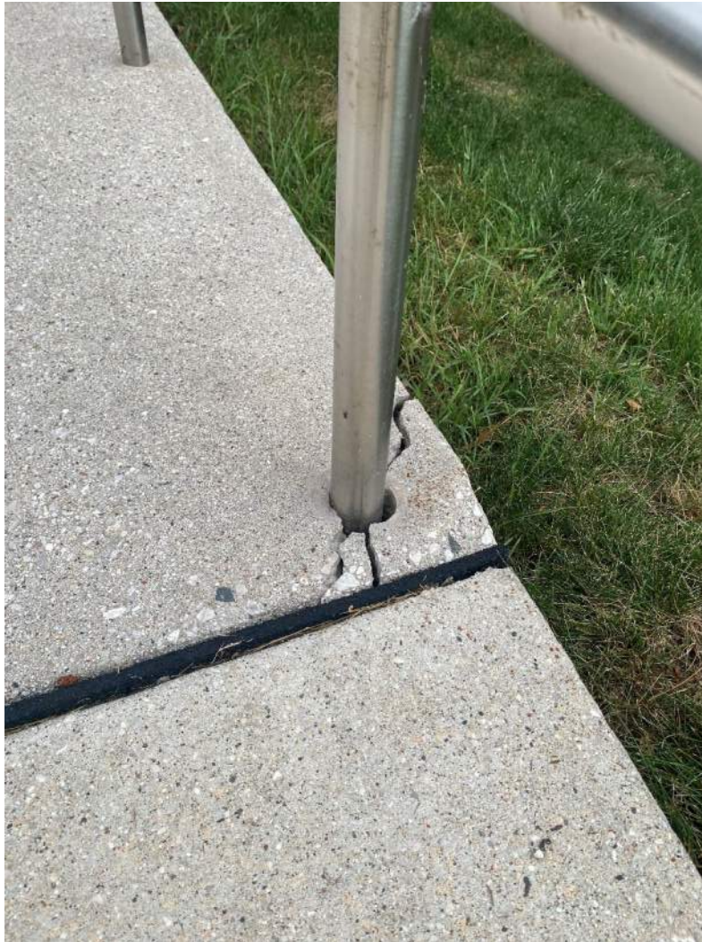
Figure 20: Cracking concrete at railing poles on front concrete ramp.
