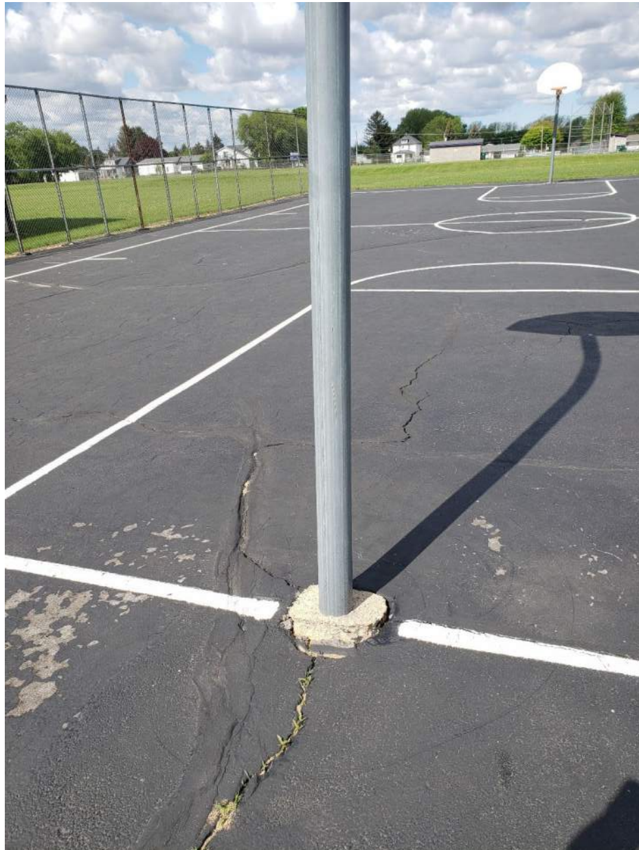
Figure 25: Basketball court with alligator and transverse cracking
