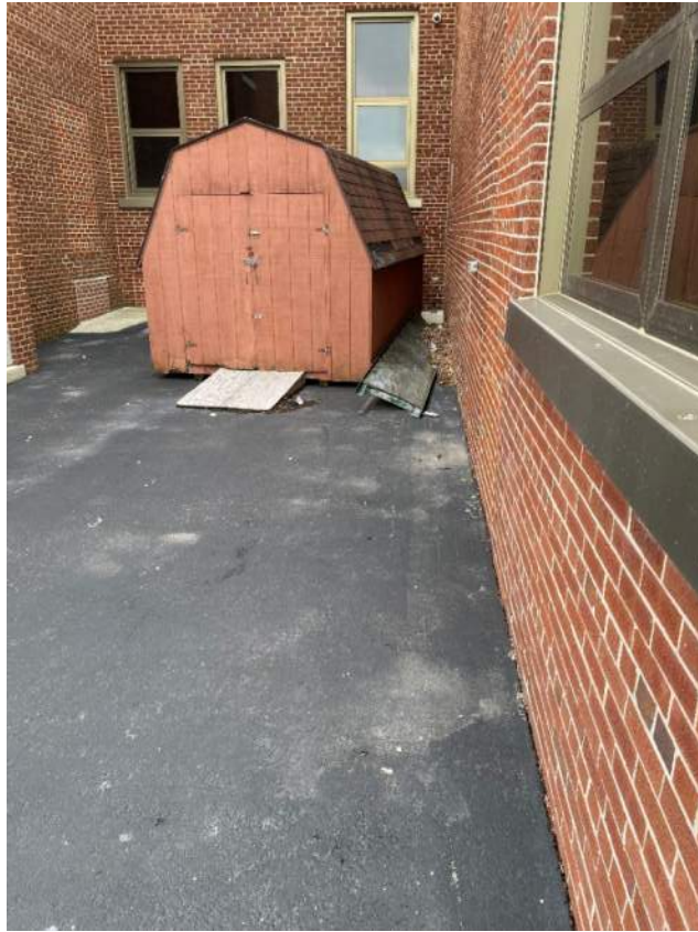
Figure 44: Deteriorating shed in back play yard.
