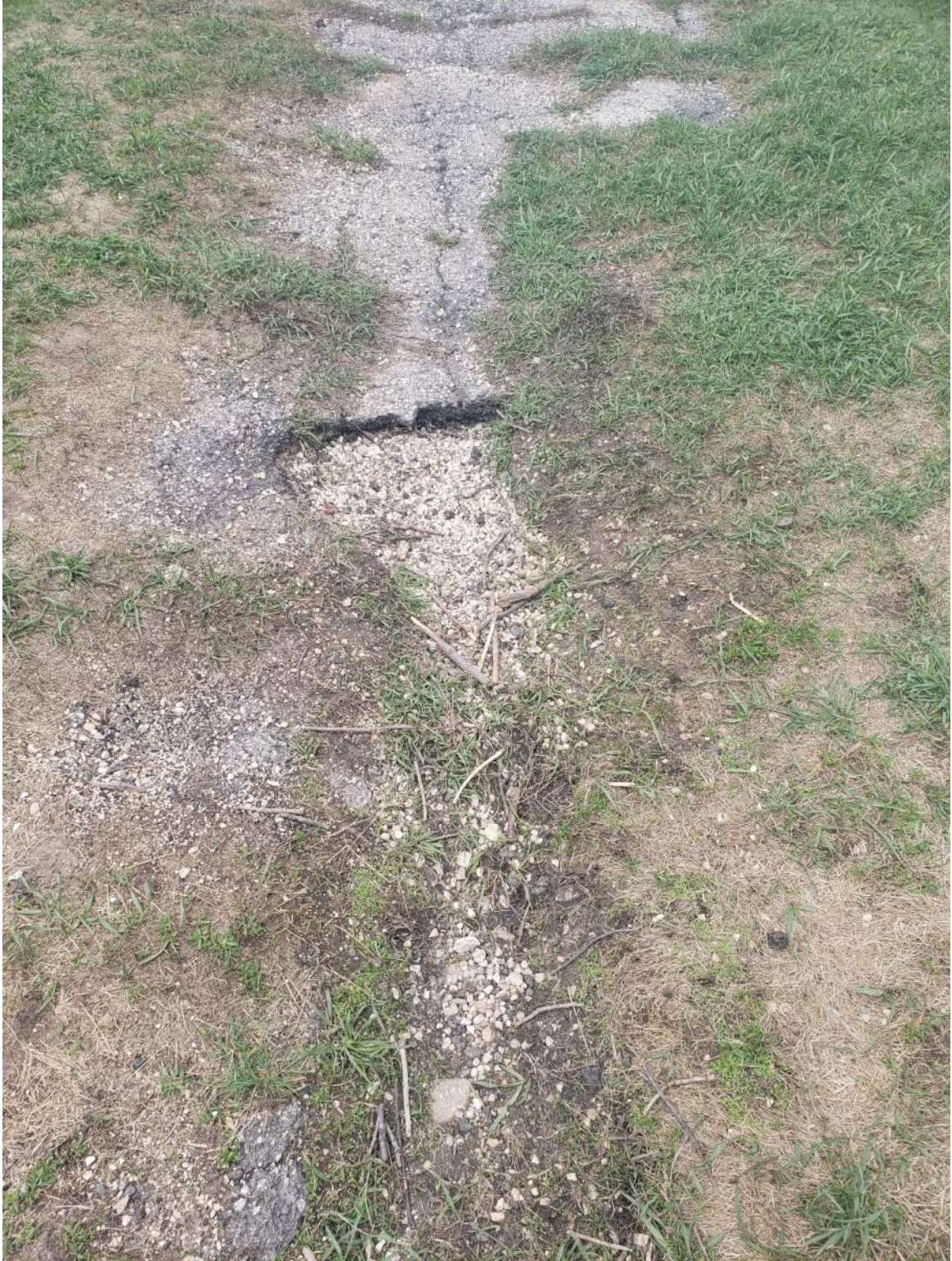
Figure 16: Swale near NE portion of play yard in poor condition
