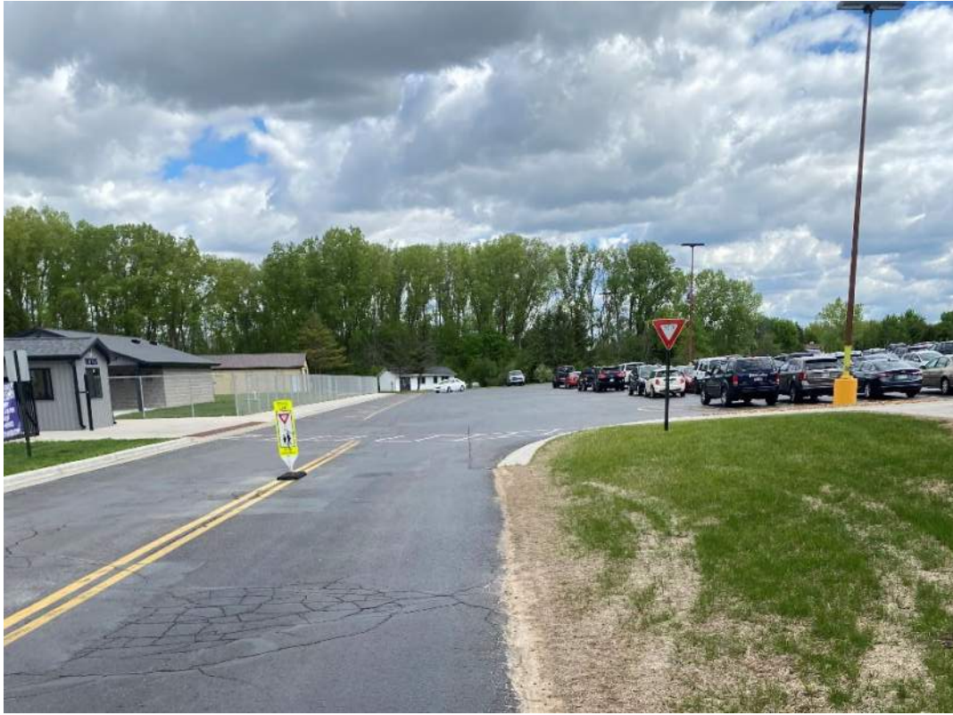
Figure 12: Alligator Cracking on north portion of Access Drive.
