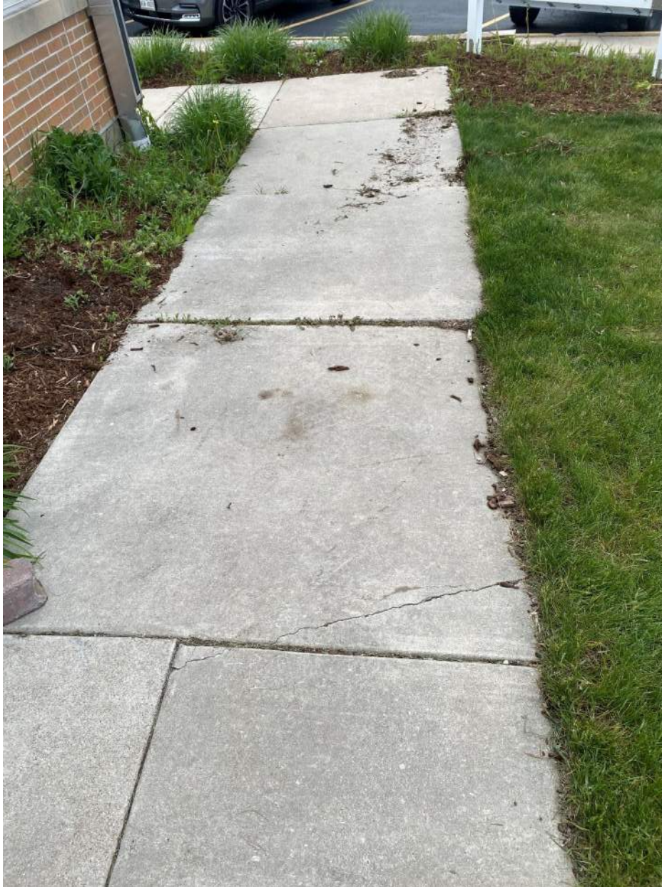
Figure 17: Cracked and uneven sidewalk around greenhouse
