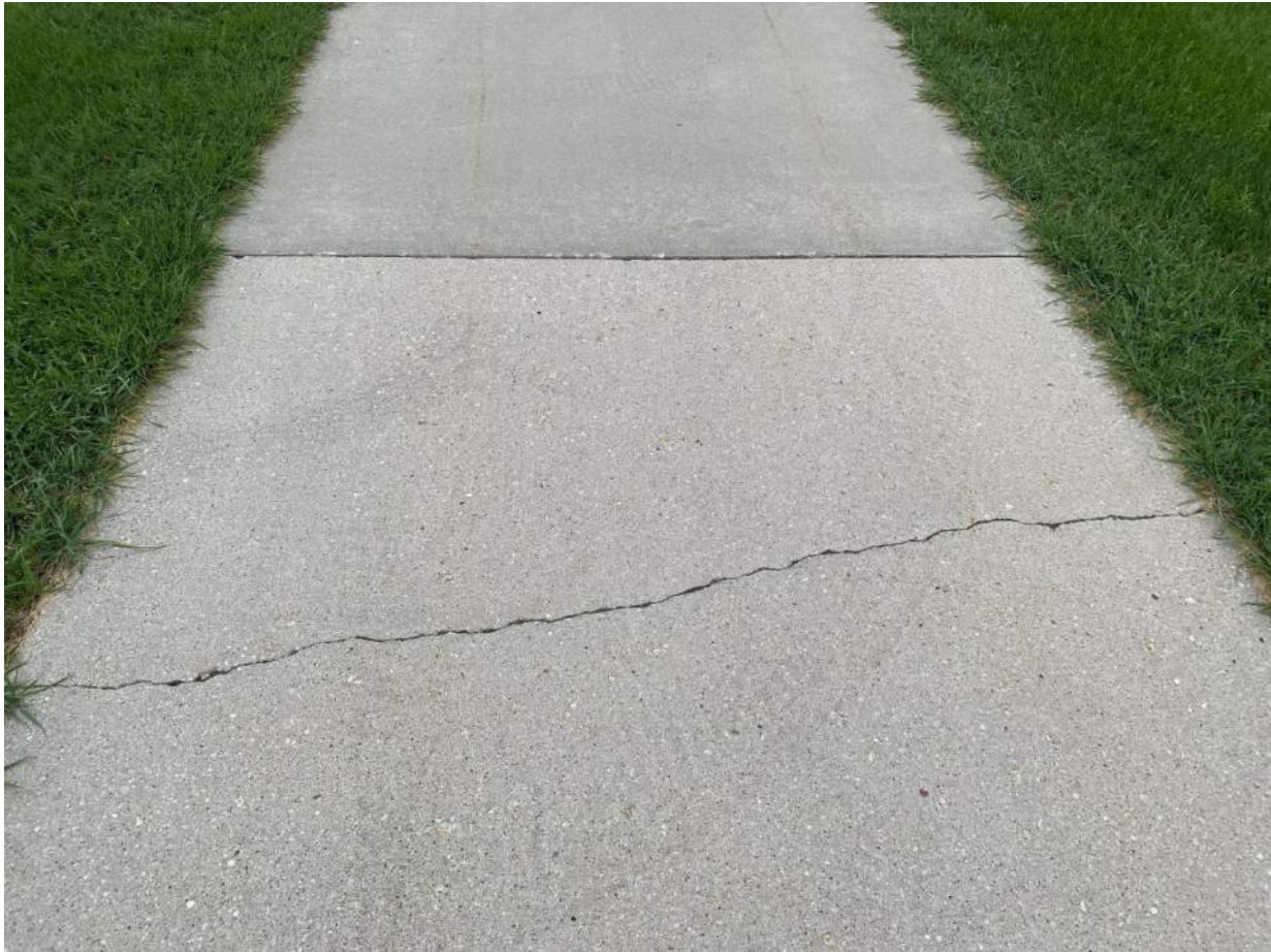
Figure 16: Diagonal crack in front center west sidewalk.
