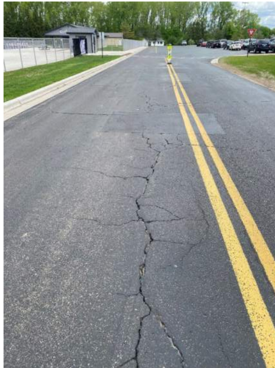
Figure 13: Longitudinal and Transverse Cracking on north portion of Access Drive.
