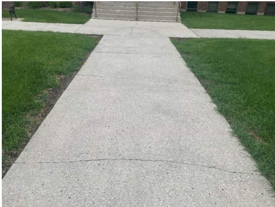
Figure 10: Horizontal cracking in front center east Sidewalk.
