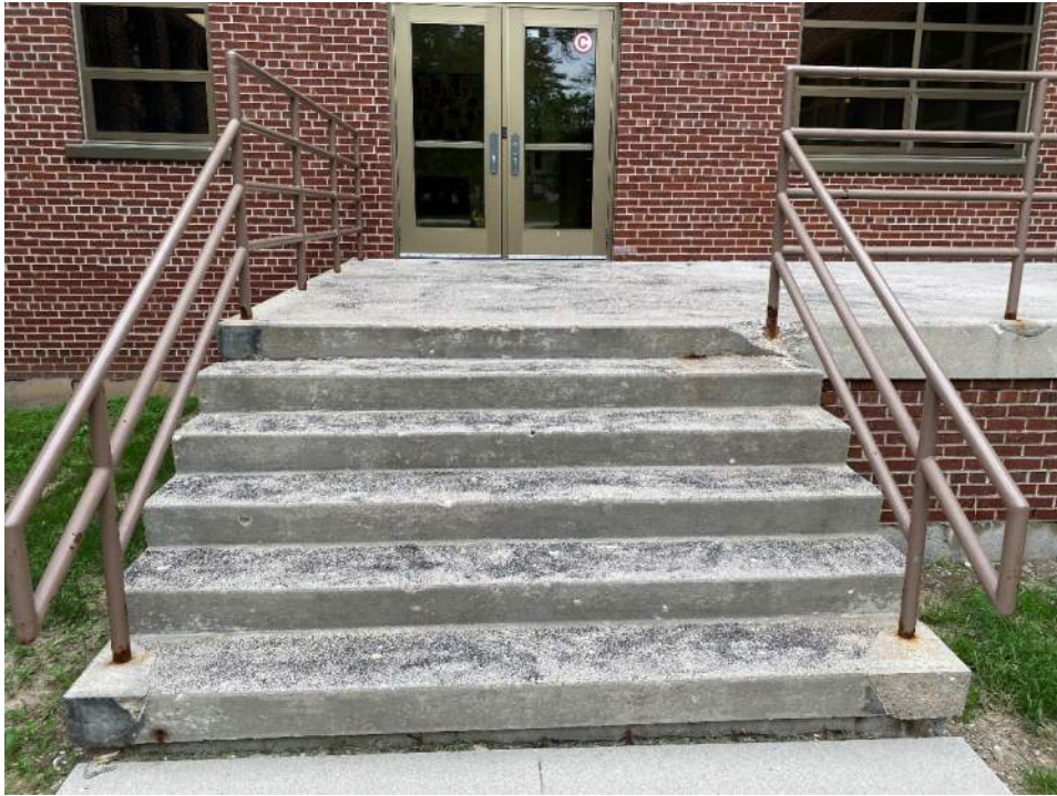
Figure 4: Front east stairs in poor condition.
