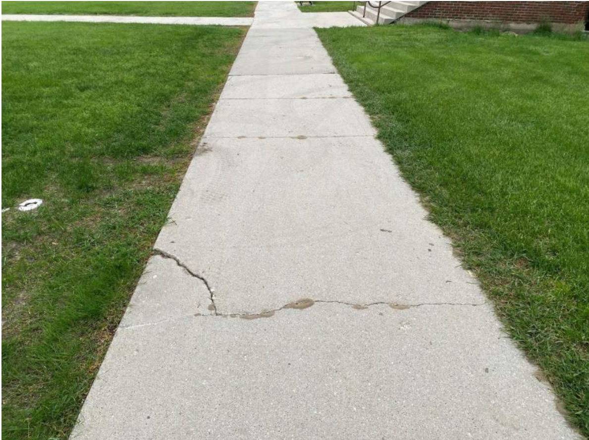
Figure 6: Cracking in east to west sidewalk.
