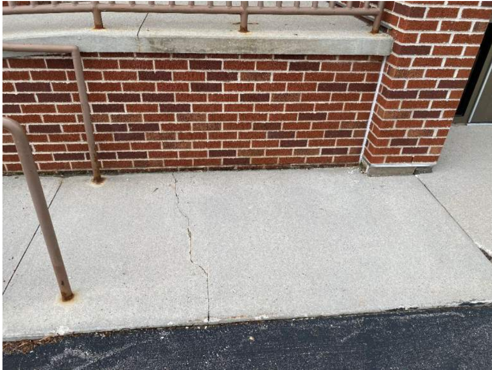
Figure 40: Cracked slab at landing of back concrete ramp.
