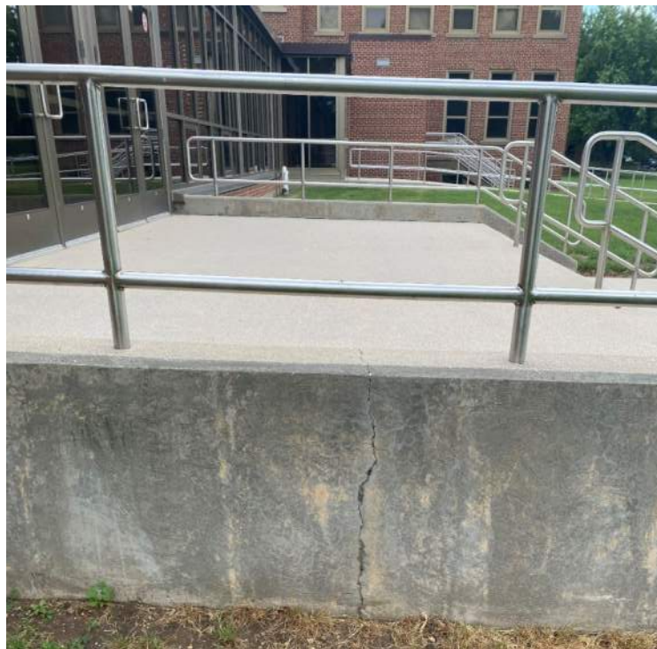
Figure 24: Another foundation crack on front west stairs.
