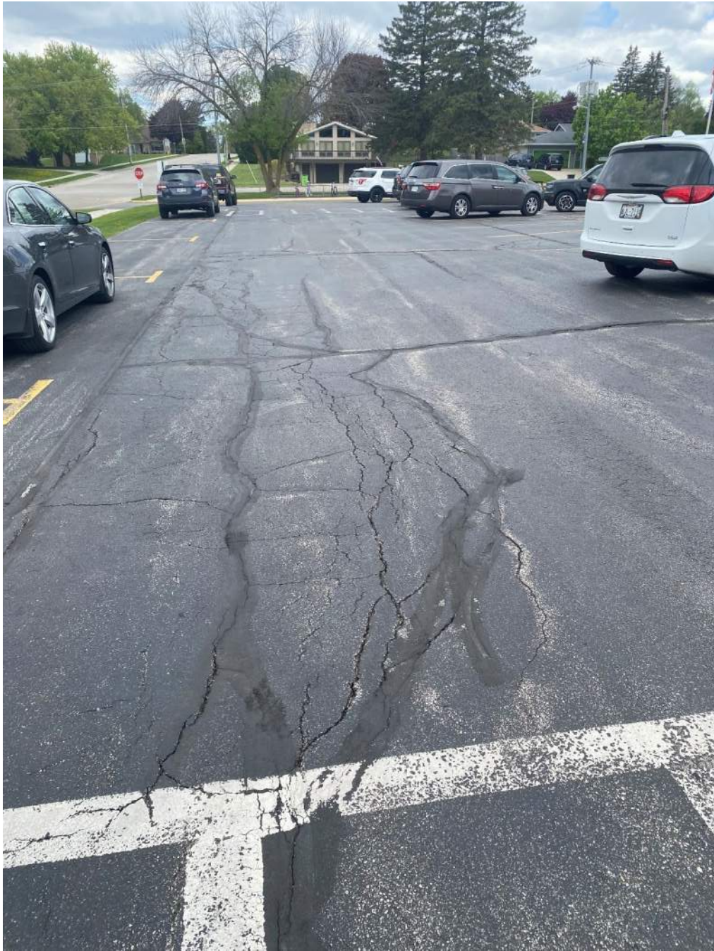
Figure 9: South parking lot cracking
