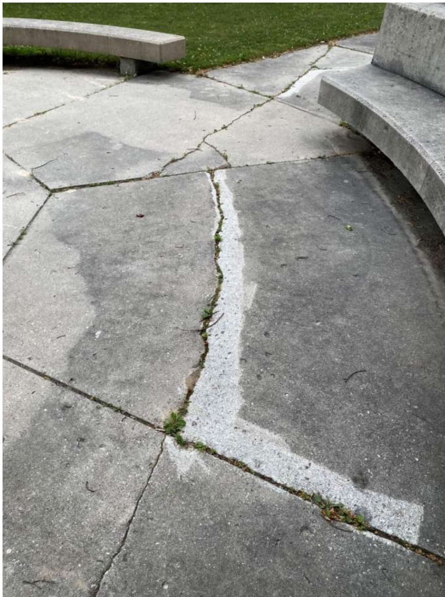
Figure 39: Cracking and settling concrete in courtyard.
