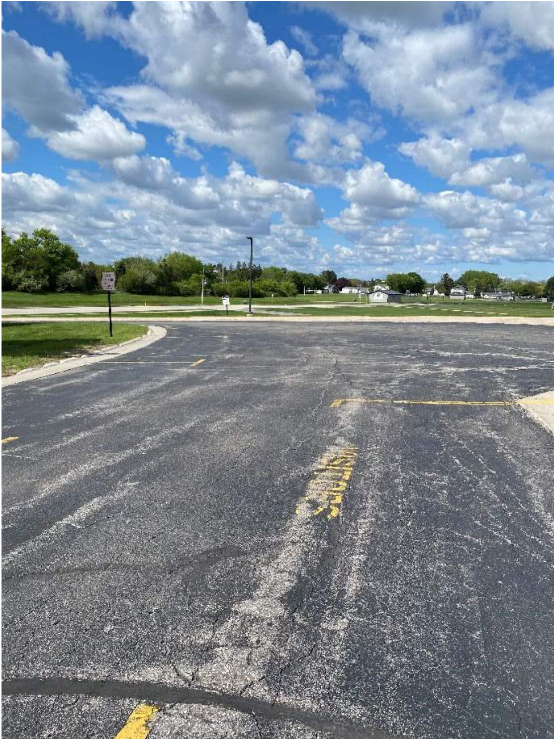
Figure 3: Faded pavement markings in Bus/Visitor Parking Loop.
