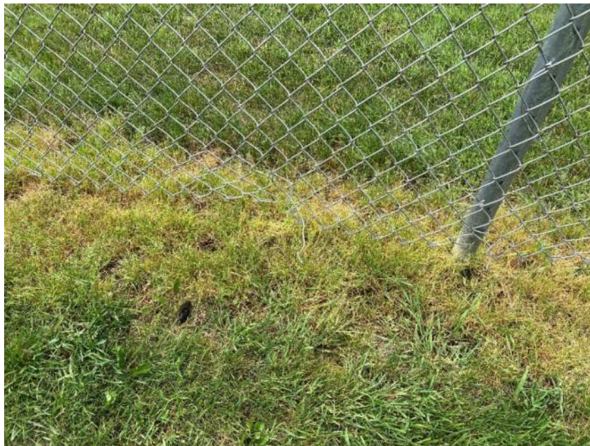
Figure 55: Exposed wire on bottom of fence surrounding climbing equipment.
