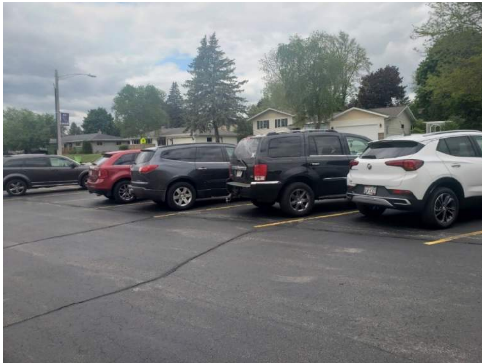
Figure 4: Transverse crack in West parking lot.
