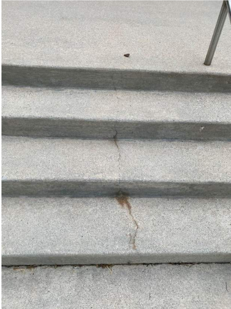
Figure 25: Crack on stairs of front west stairway.
