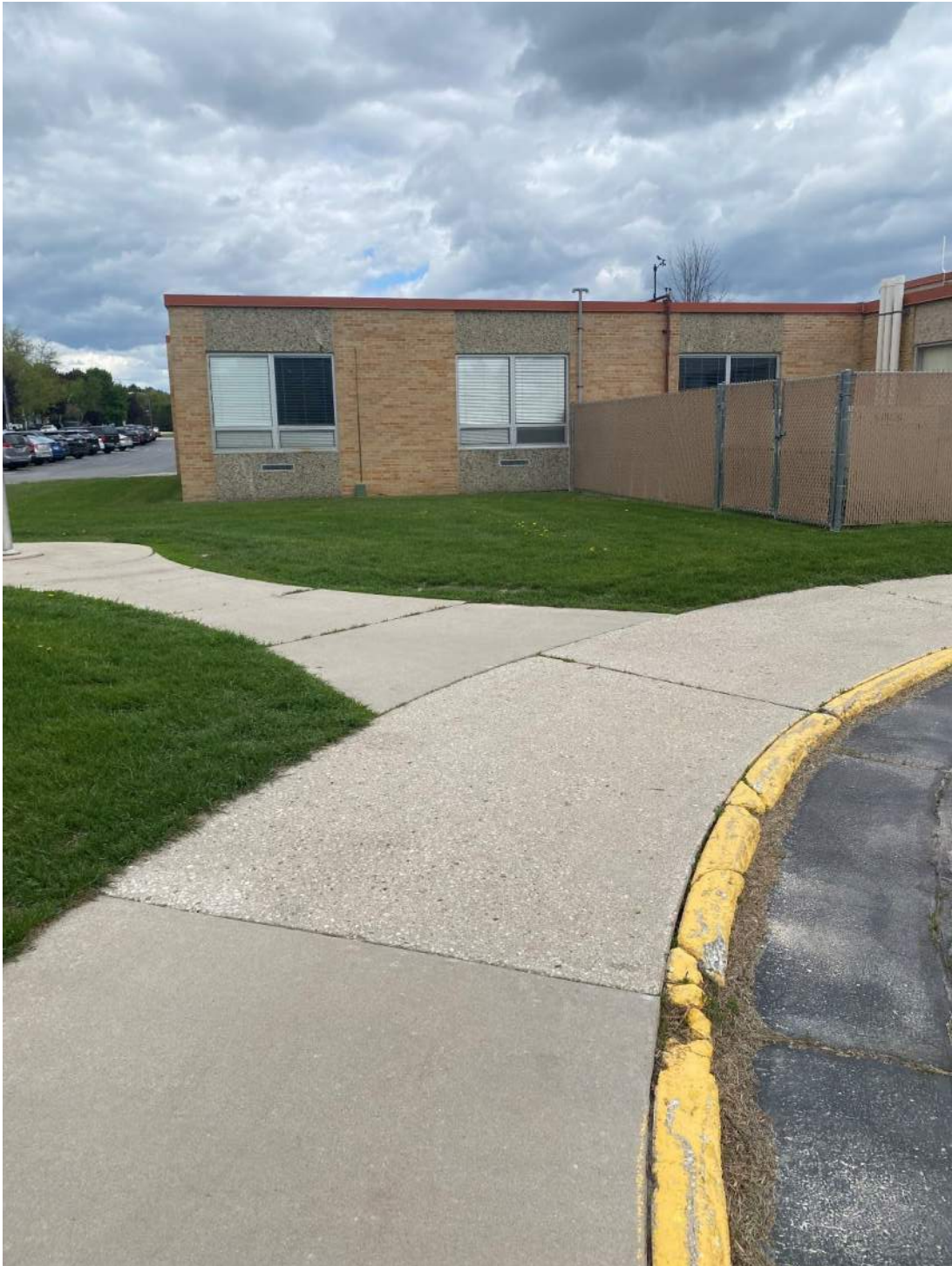
Figure 11: Cracked and deteriorating curb in north-west corner of south parking lot
