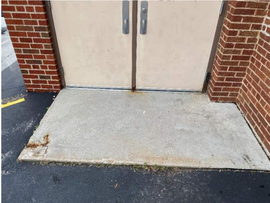
Figure 43: Deteriorating concrete stoop in back play yard.
