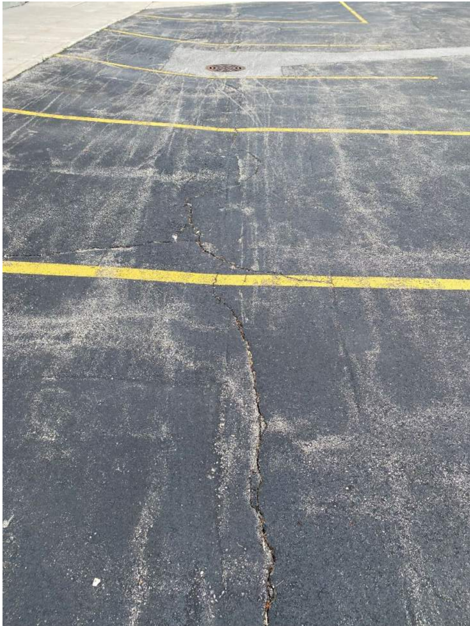
Figure 75: Longitudinal cracking in northwest parking lot.
