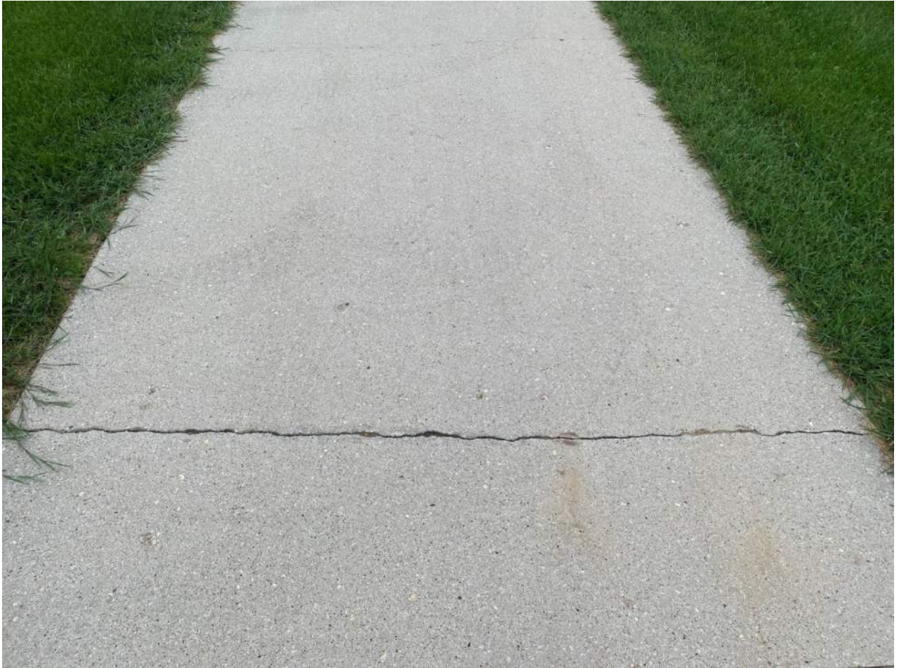
Figure 15: Horizontal crack in front center west sidewalk.
