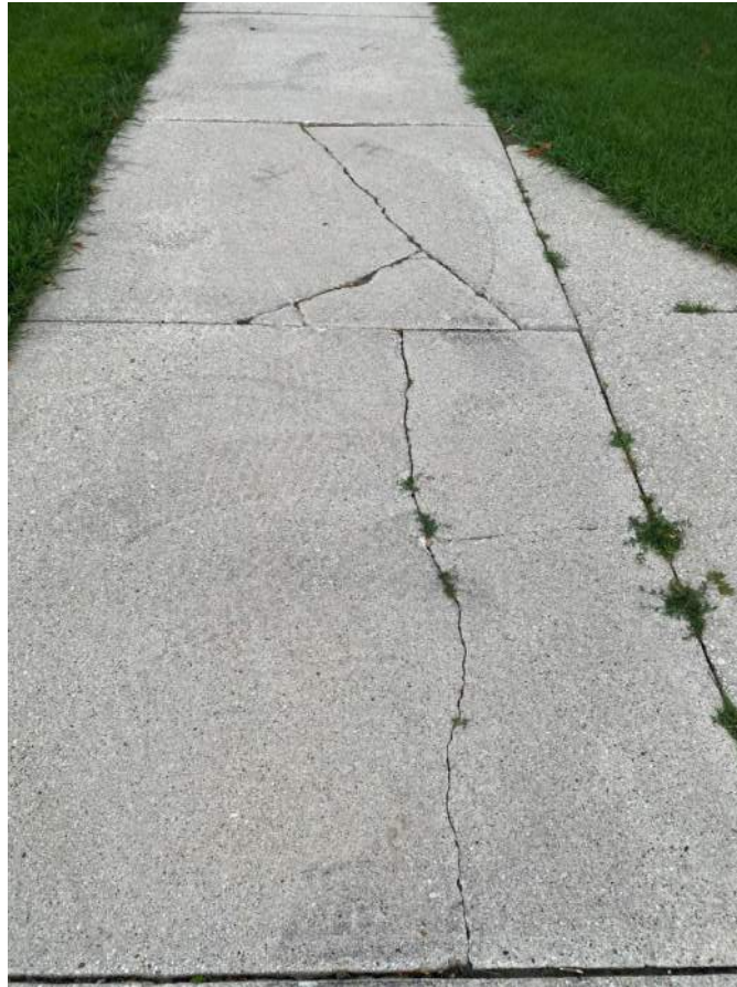
Figure 26: Severe cracking in front west sidewalk.
