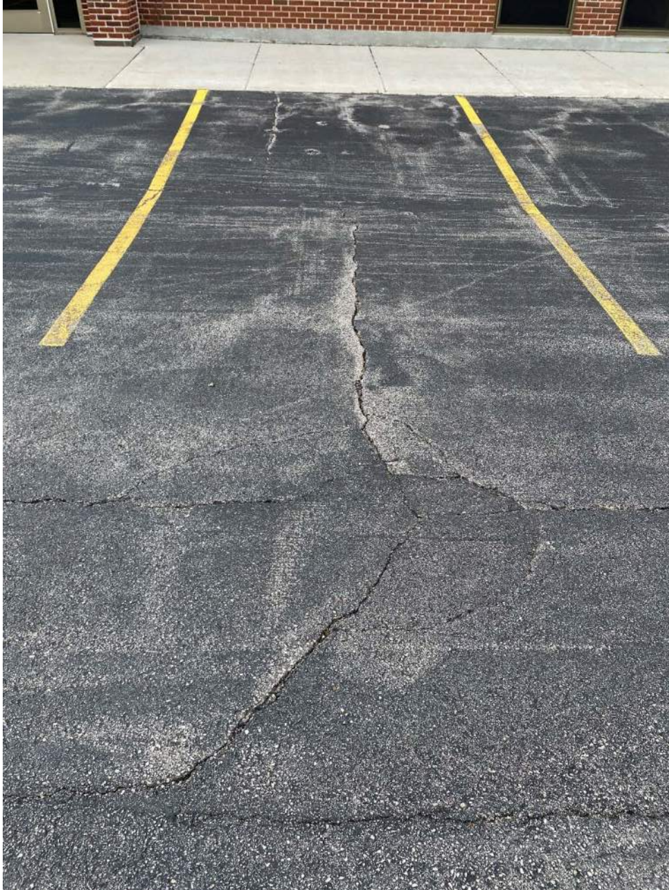
Figure 37: Cracking and settling in northwest parking lot.
