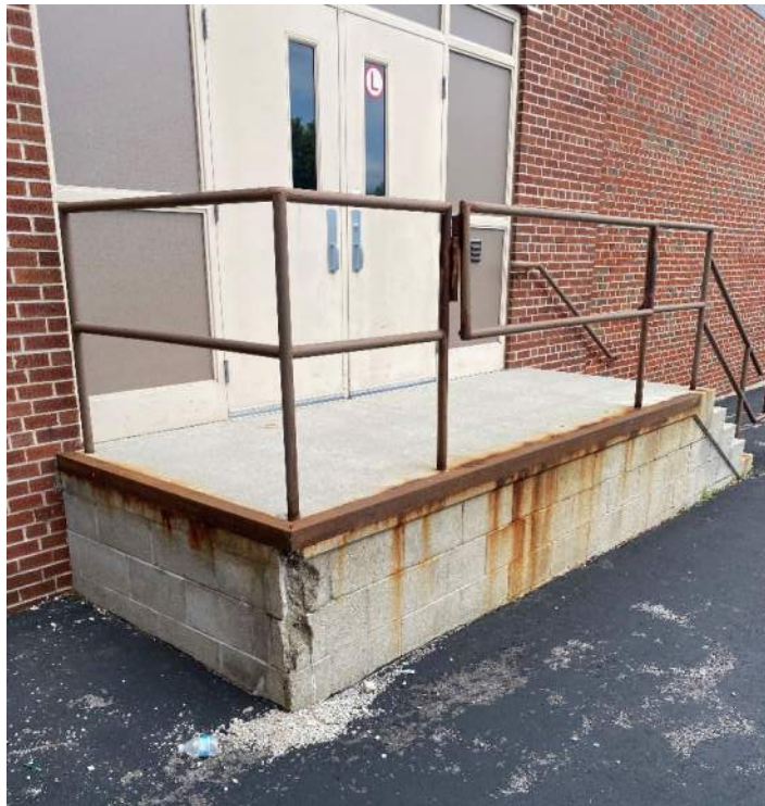
Figure 46: Concrete stair in back play yard in poor condition.
