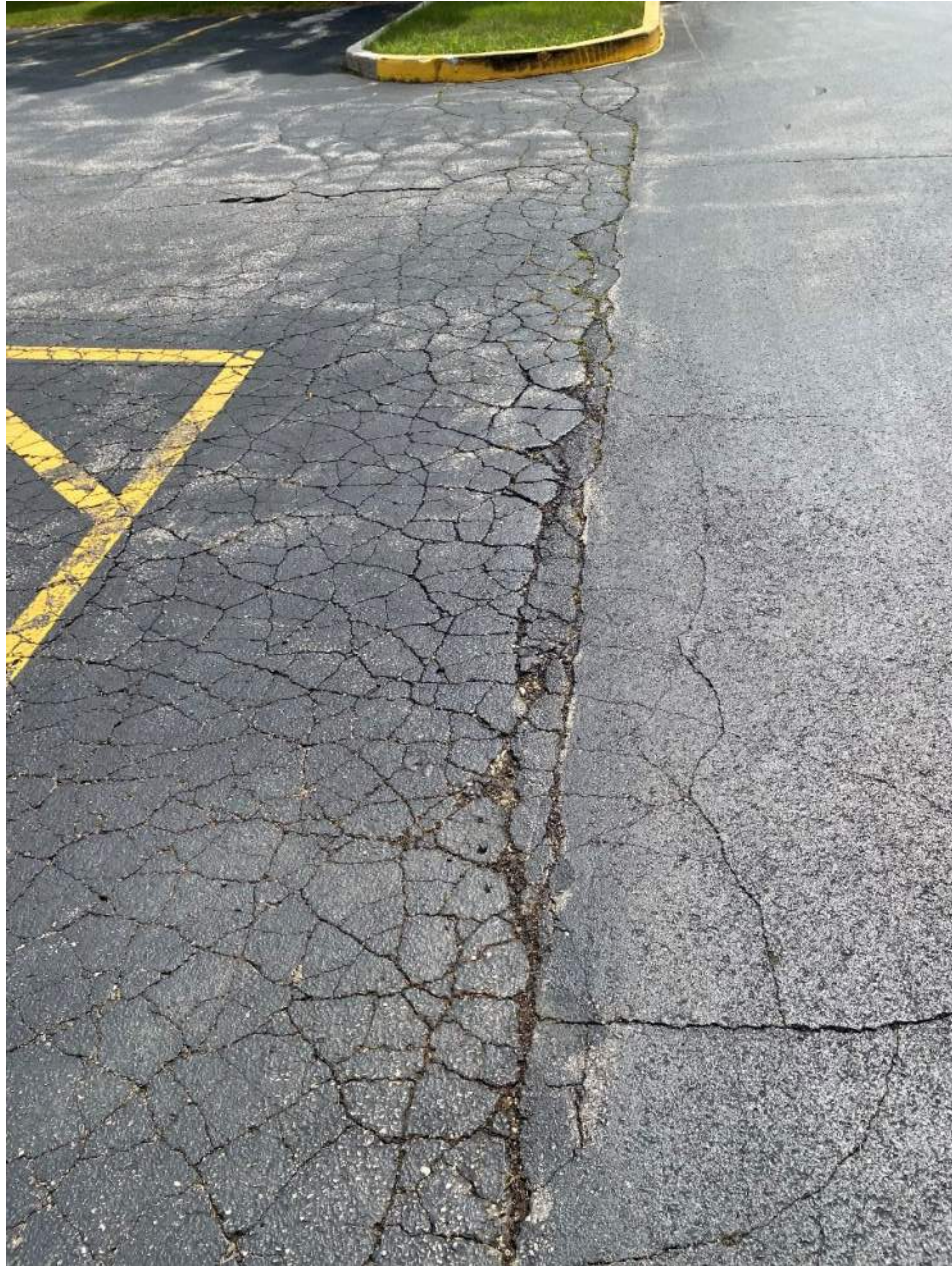
Figure 53: Alligator cracking near entrance to back northeast parking lot.
