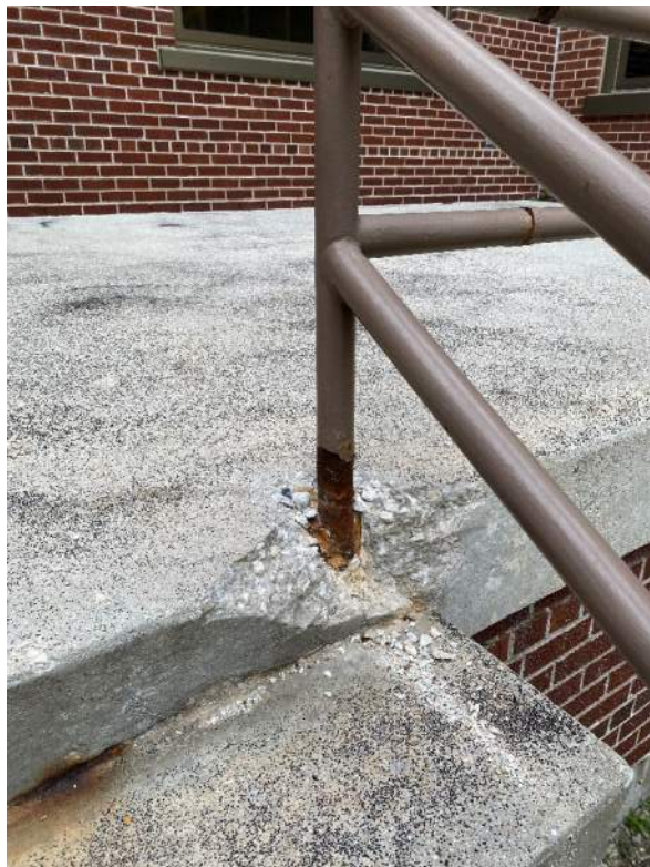
Figure 5: Concrete deterioration at railing post on Front East Stairs.
