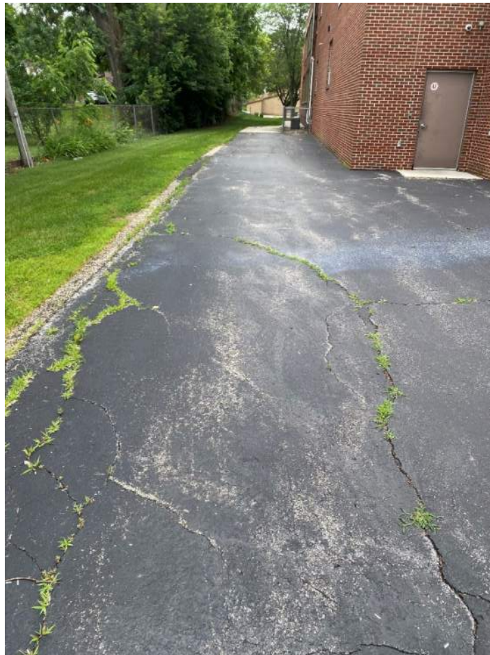
Figure 59: Longitudinal, transverse and block cracking in asphalt on east side of school.
