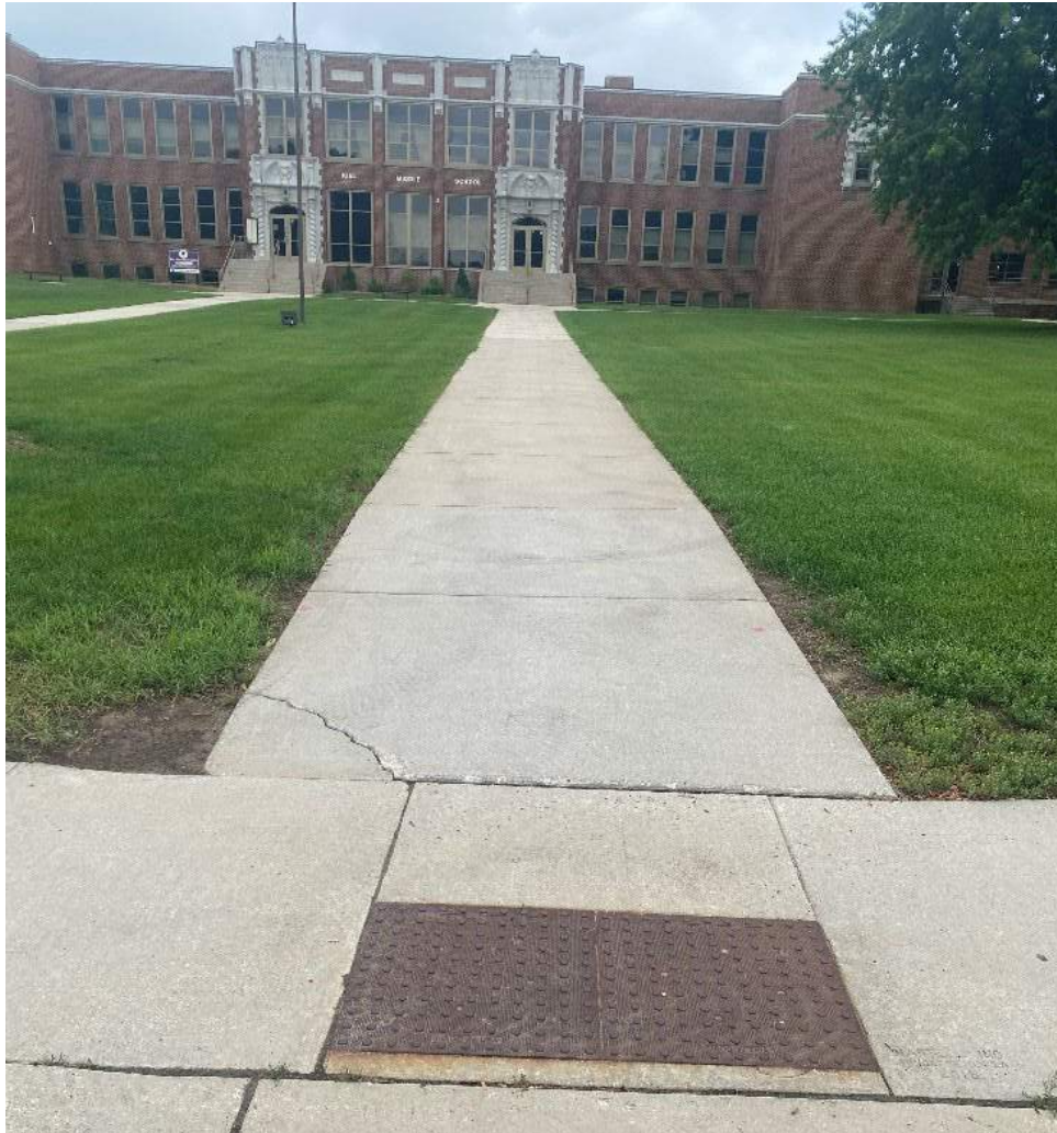
Figure 11: Corner of concrete sidewalk slab cracked off at south slab of center east sidewalk.
