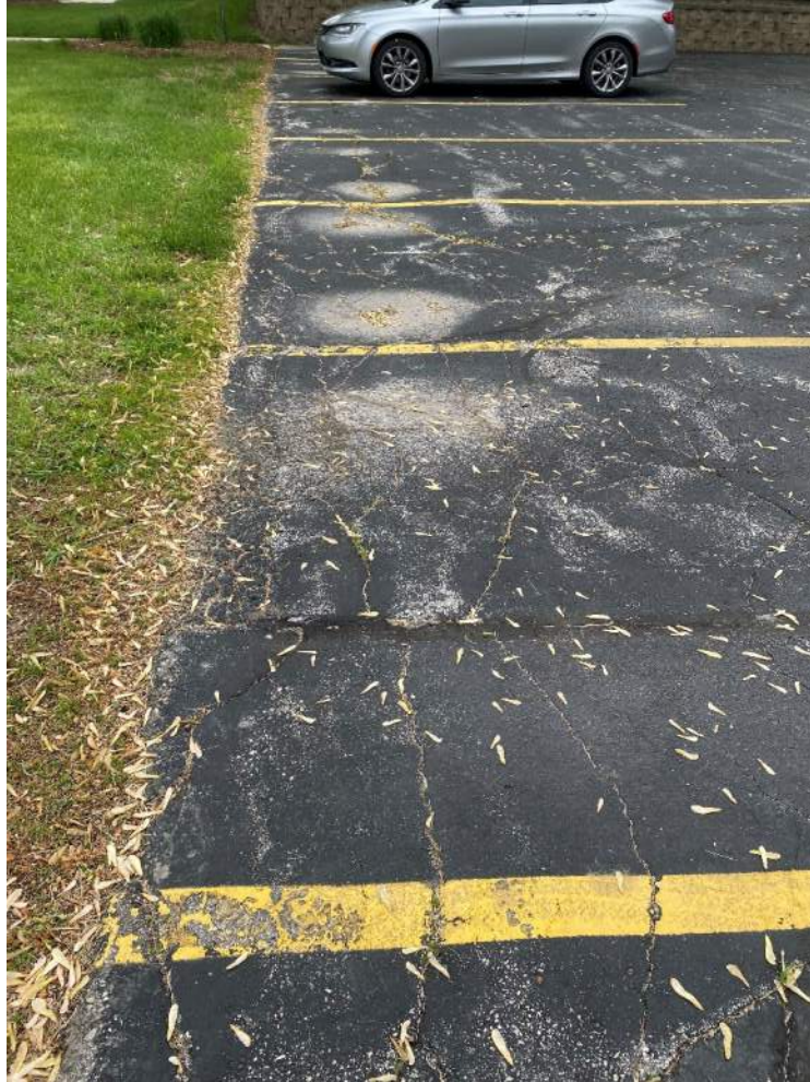
Figure 3: Pavement settling occurring in southeast parking lot.
