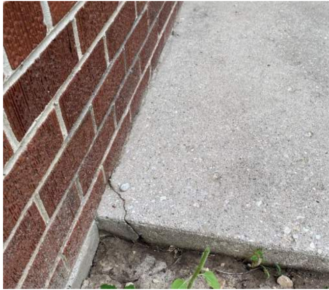
Figure 30: Corner cracked off concrete slab at door on west side of school.
