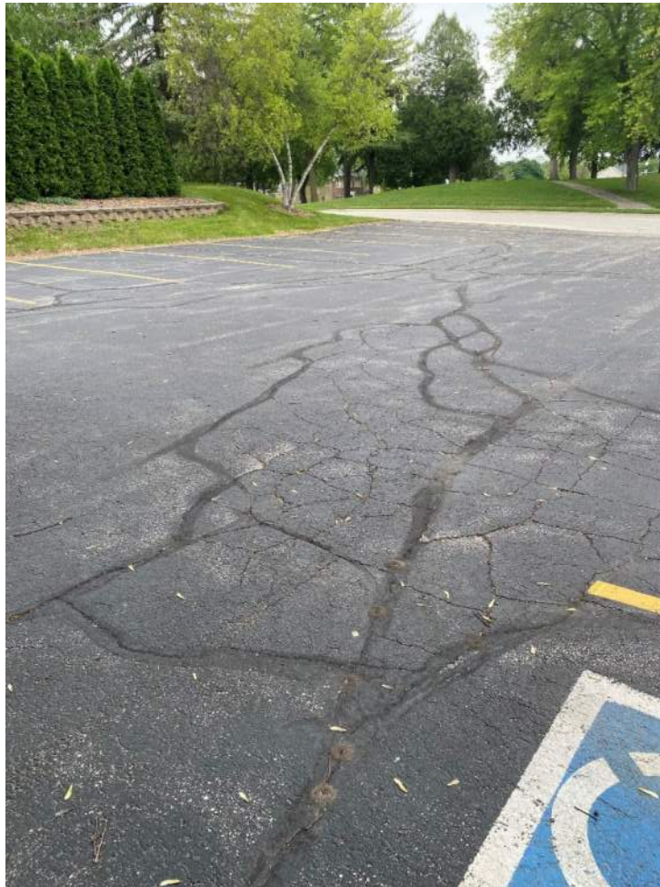
Figure 2: Block, transverse, and longitudinal cracks in southeast parking lot.
