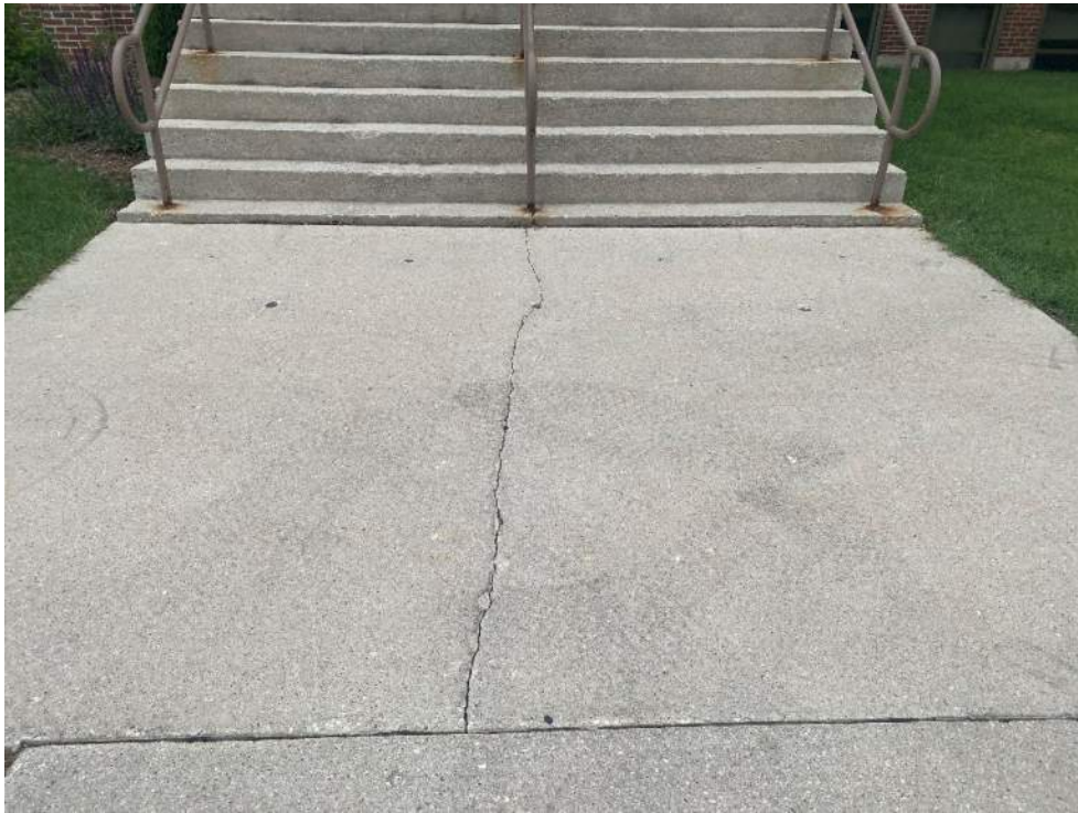
Figure 9: Vertical crack in concrete slab at bottom of front center east stairs.
