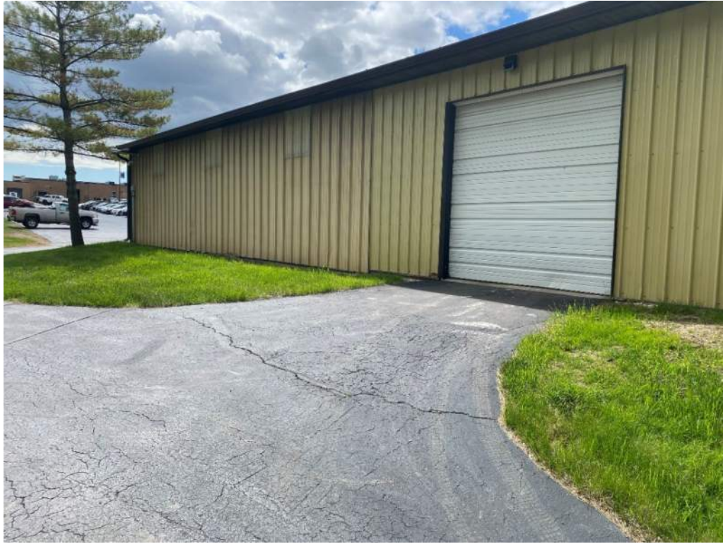
Figure 15: Pavement cracking near shed in northwest corner of Student Parking Lot
