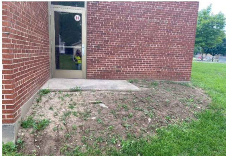
Figure 31: Concrete slab and surrounding grass in good to fair condition on west side of school.
