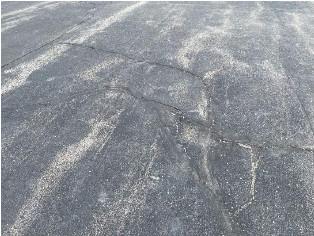
Figure 24: Cracks in play area surface
