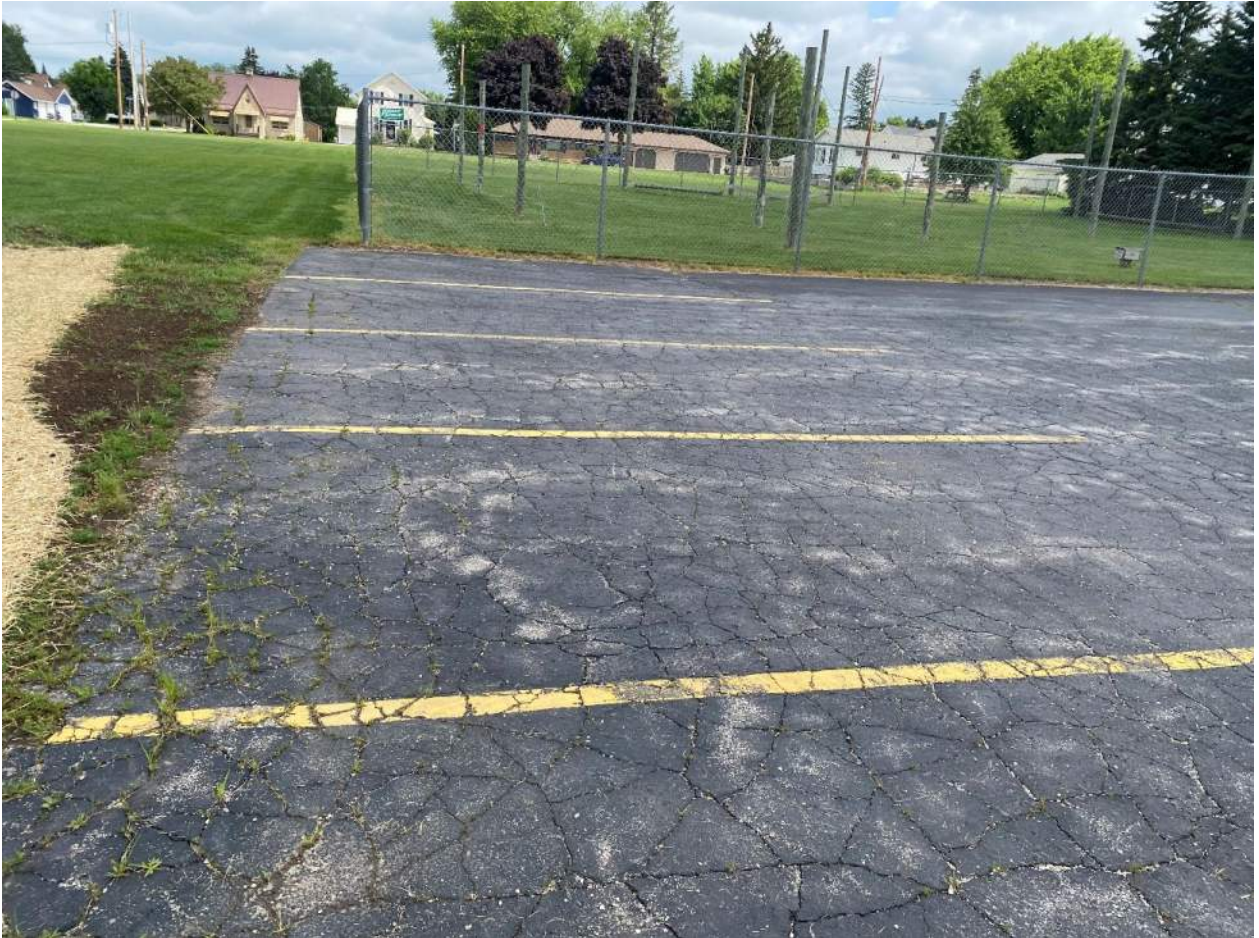
Figure 52: Northeast parking lot covered in alligator cracking.
